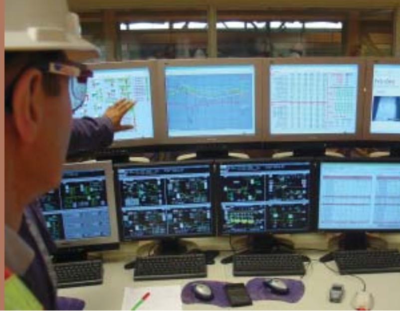
Control room at Antamina concentrator, Peru.
