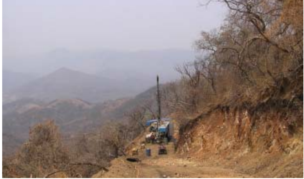
Drilling at Morelos property, Mexico. Results in 2003 include 40 g/t gold over 9 metres.
