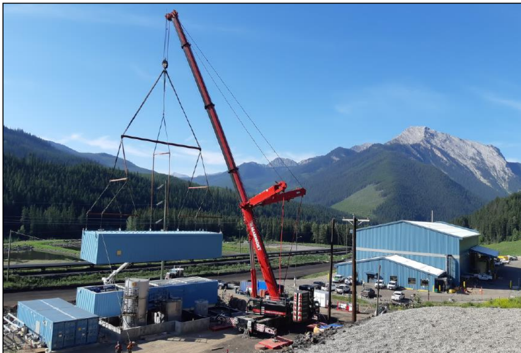
Figure 2-6 Summer 2018 Placement of the Advanced Oxidation Process at the West Line Creek Active Water Treatment Facility
