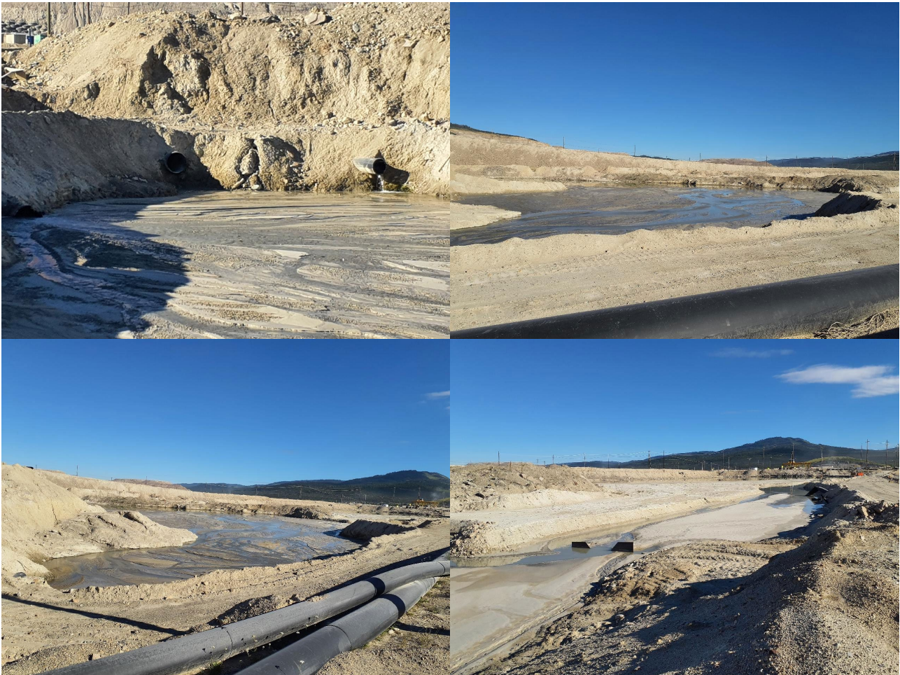
Photo I-1 7-Day Pond TSF. Two inflow pipes observed: one pipe discharging clear water at the time of the site visit (SDP-2022-01, SDP-2022-02 and SDP-2022-03)
