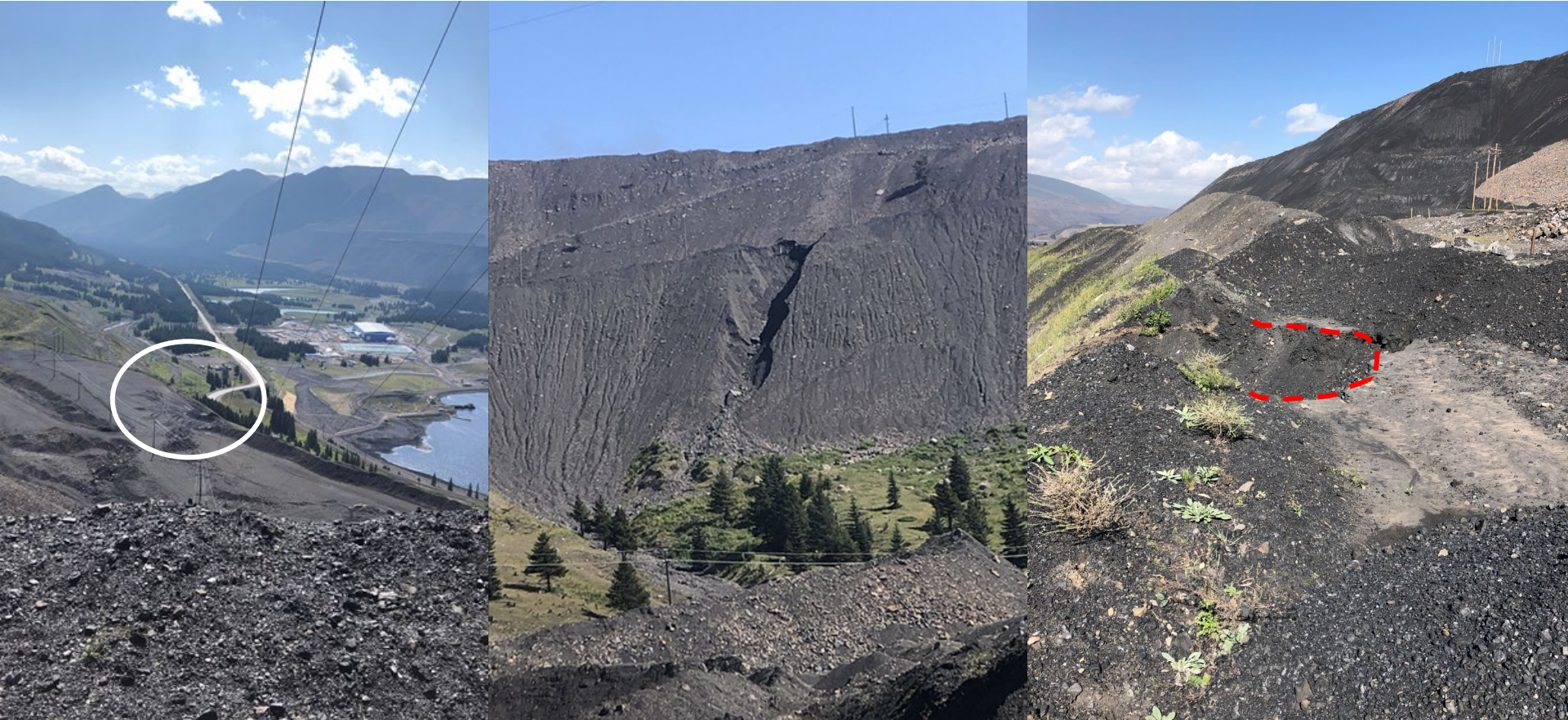
Blake spoil - Erosion channel and loss of berm on western lift due to surface water. Run out of coal rejects onto 1,730 lift of Kilmarnock / Toe Berm spoil
