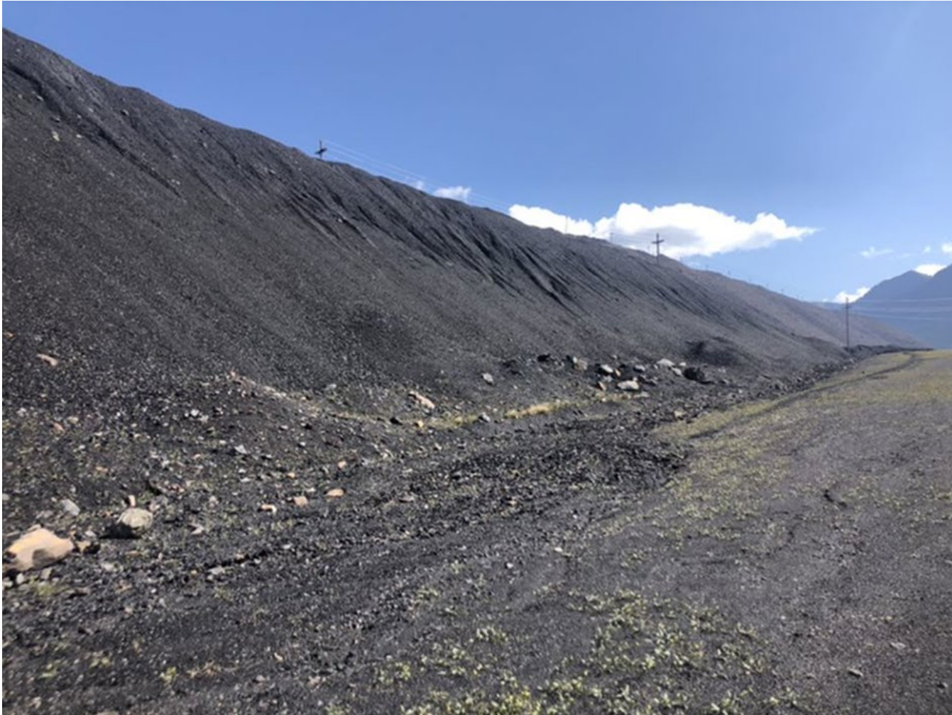
Blake spoil - Upper lift with minor erosion rilling, looking south
