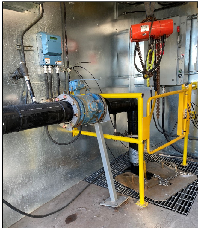
Photograph 14: Seepage collection sump pumphouse
