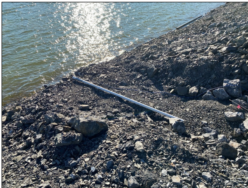
Photograph 15: Piezometer cable extension at upstream slope
