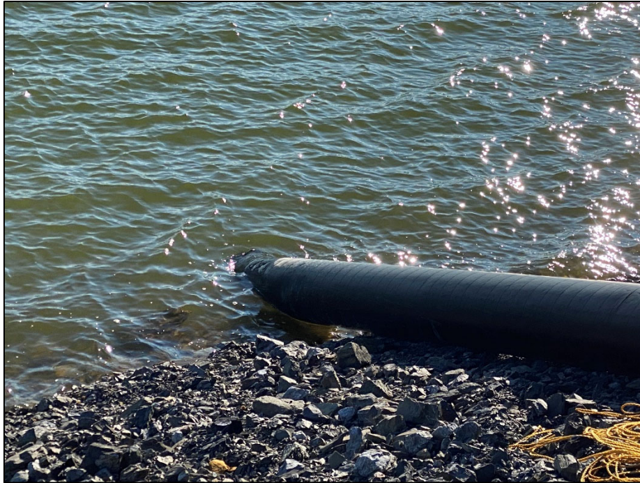
Photograph 13: Seepage return discharge pipe
