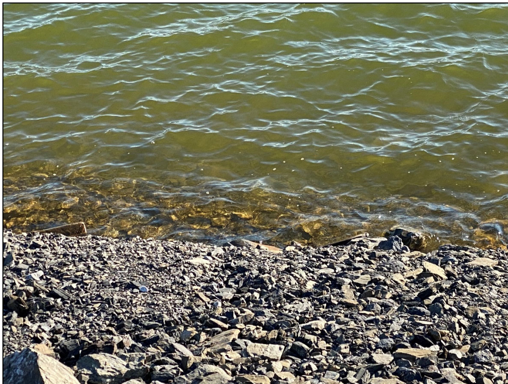
Photograph 07: Wave erosion on upstream slope
