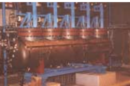
The CESL hydro-metallurgical autoclave dissolves the copper minerals into a solution
