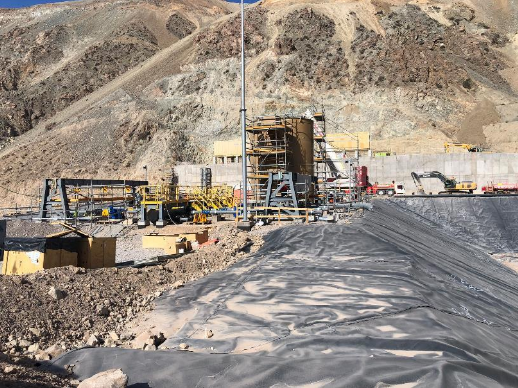
Central berm & pumping infrastructure
