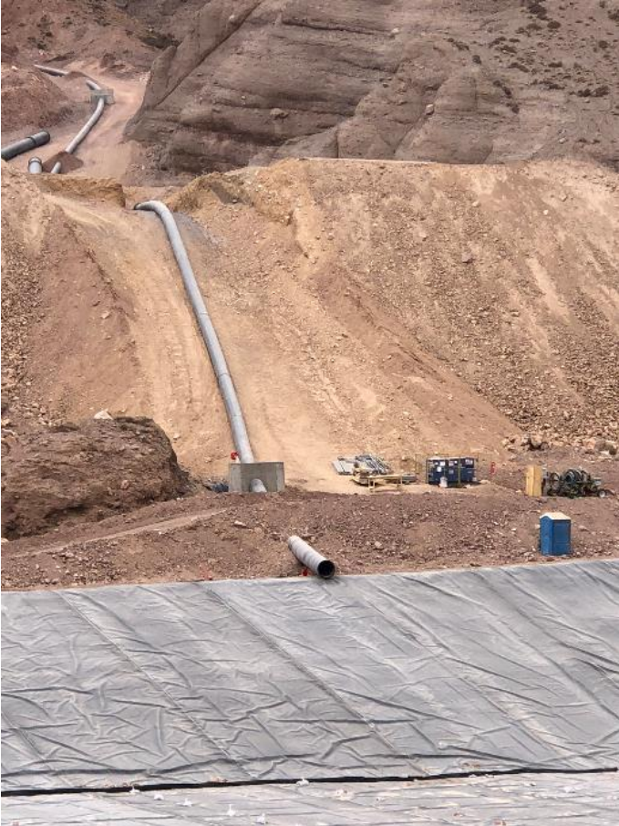
Outlet of emergency discharge pipeline
