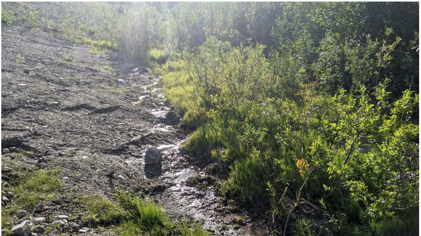
Photo ND-08: Downstream toe of the North Dam looking west at the base of the erosion gully repair area.
