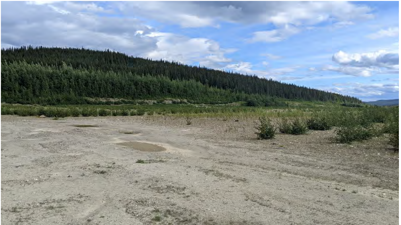
Photo TC-01: North Dam crest and tailings cover south of the erosion gully repair area.
