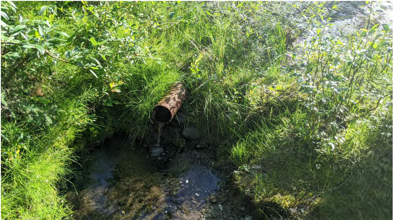
Photo ND-06: MH-02 flow monitoring pipe.
