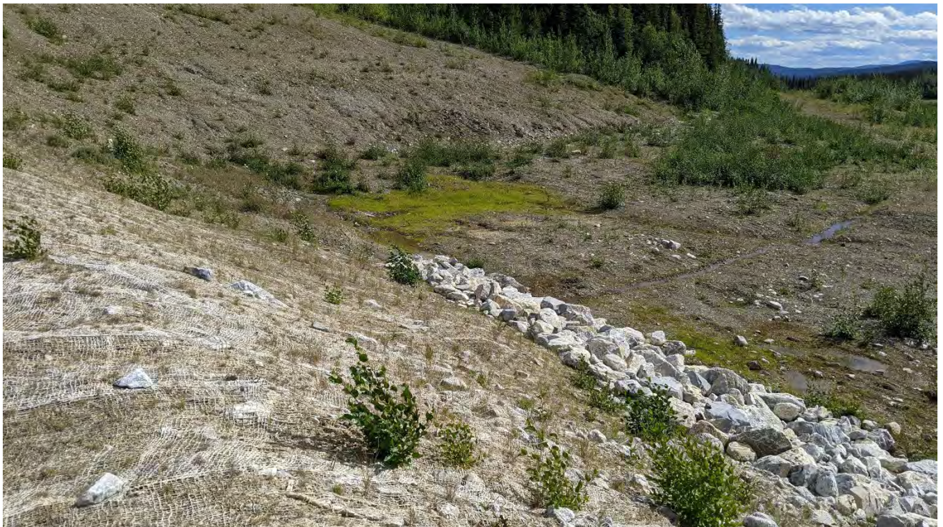
Photo SRS-06: Downstream face of the SRS on the east side of the spillway looking southeast.
