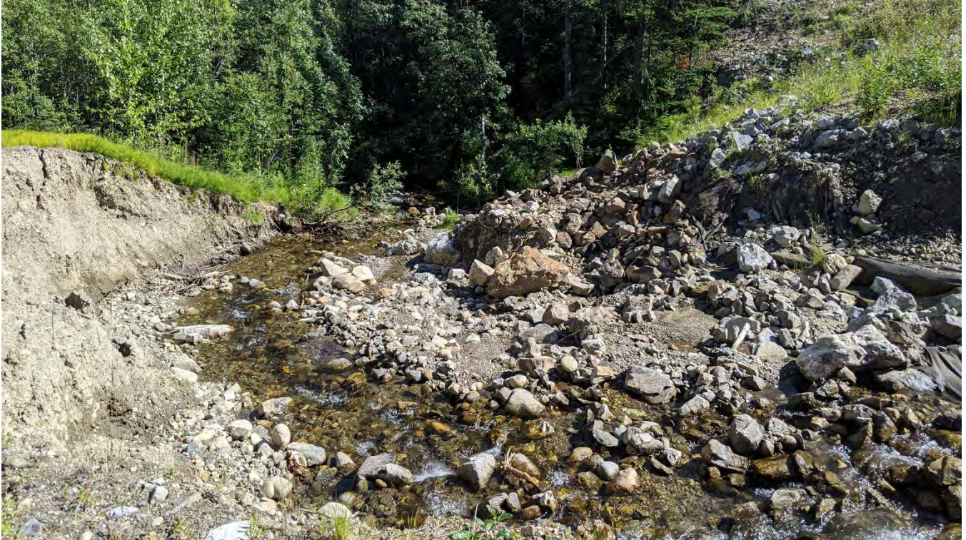
Photo NC-05: On-going channel and bank erosion at the downstream end of the lower decommissioned access road crossing of North Creek to the landfill area.
