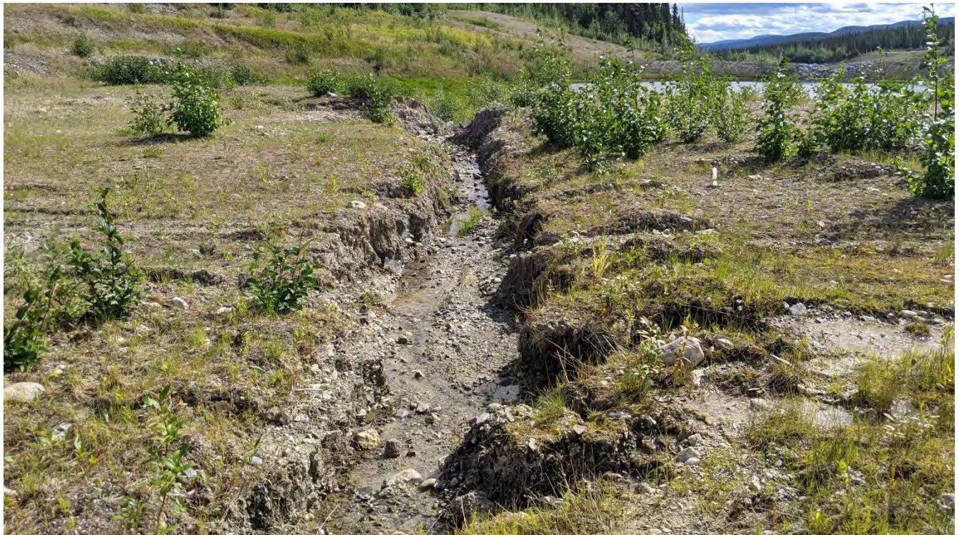
Photo TC-06: Erosion gully in tailings cover immediately to the south of the SRS Pond. Areas of exposed geotextile observed. No visible tailings observed.
