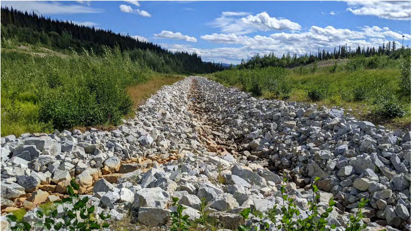
Photo DC-01: Camp Creek looking downstream at the confluence with the South Drainage Channel..
