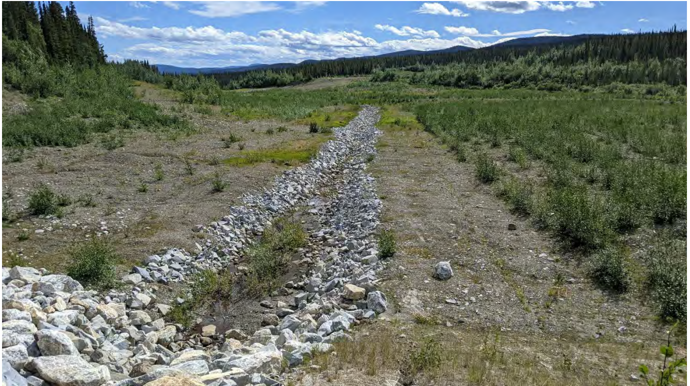
Photo DC-03: Upper end of the South Drainage Channel taken from the SRS Spillway.
