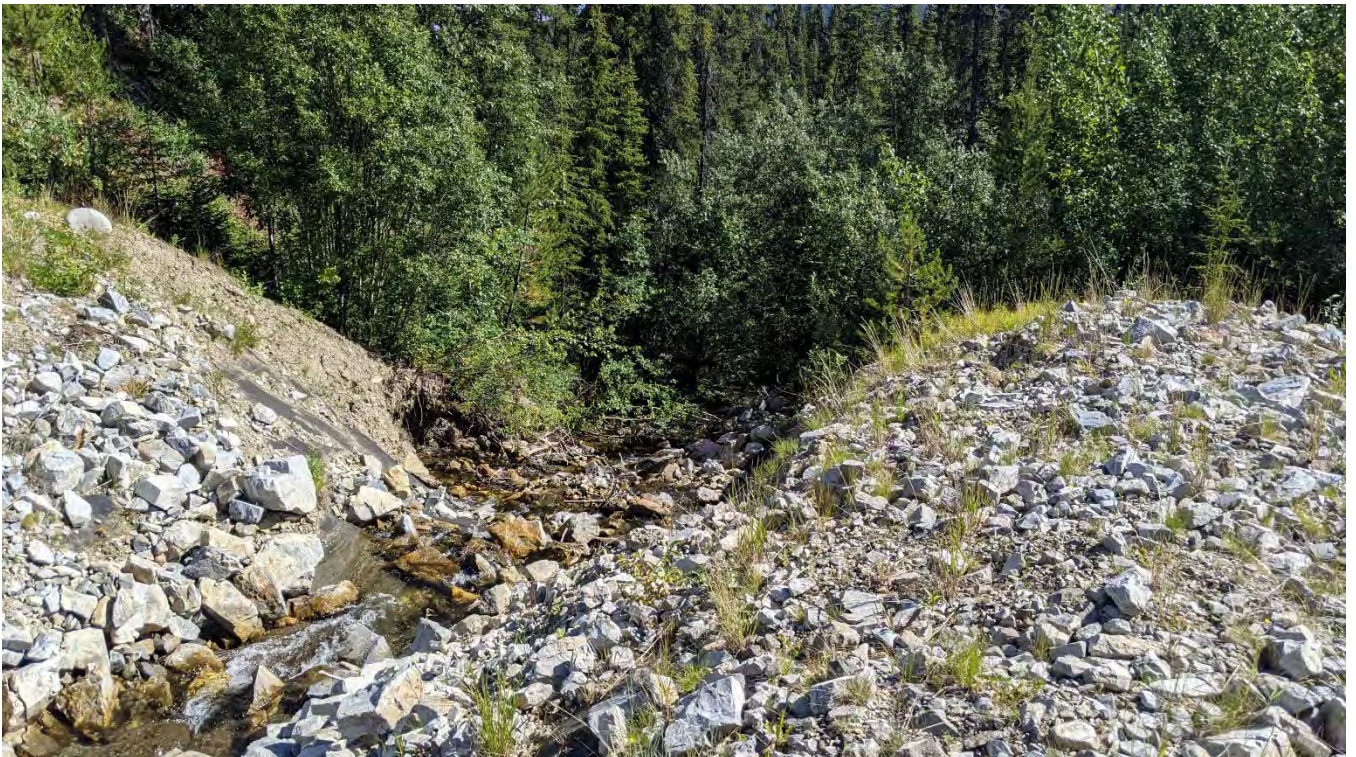
Photo NC-04: Channel erosion at the downstream end of the decommissioned North Creek Dike structure with exposed geotextile. The condition appears unchanged compared to 2021 inspection photos.
