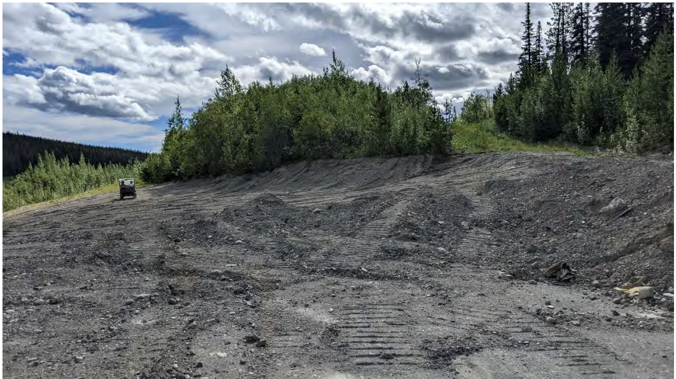
Photo ND-02: Till borrow area used for the North Dam repairs. The borrow slopes have been partially regraded and landformed.
