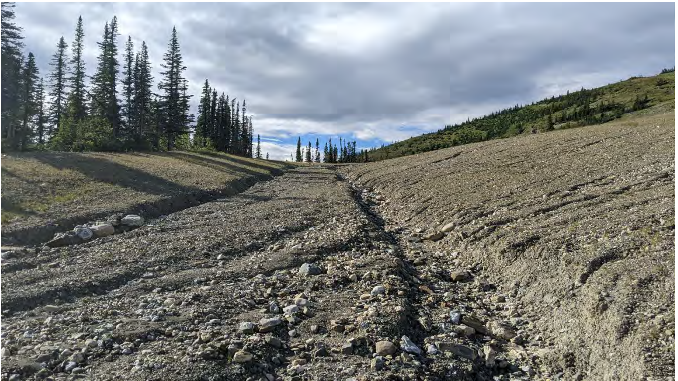
Photo WR-05: Erosion gully at the base of the Jewelbox Waste Dump looking upstream.
