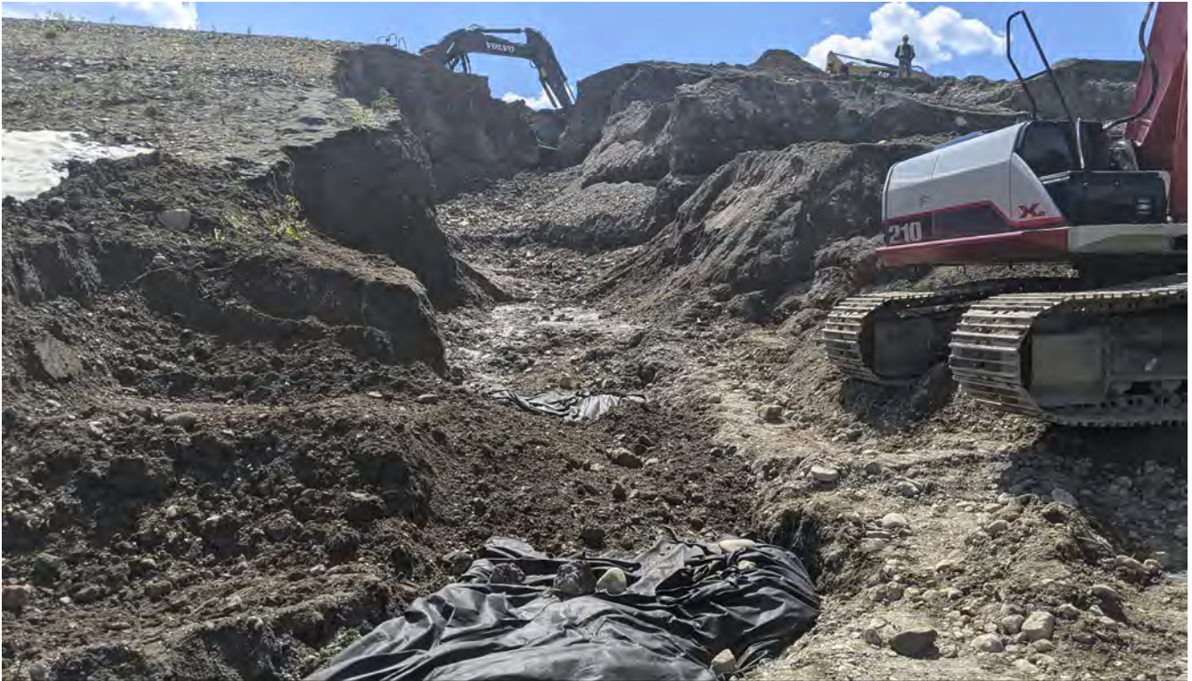
Photo 7: Sand and Gravel gully side slopes were scaled back and placed at the base of the gully (June 24, 2022).
