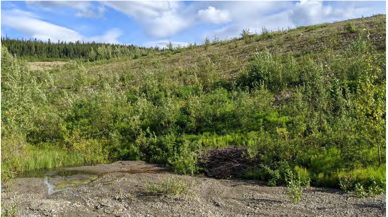
Photo ND-07: Downstream slope of the North Dam looking southeast from the base of the erosion gully repair area.
