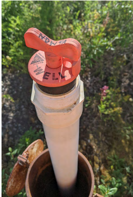
Photo ND-05: Piezometer NDW-4A downstream of the dam toe. The PVC pipe extends above the protective casing.
