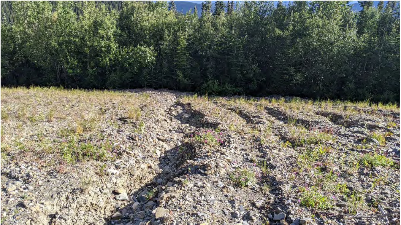
Photo WR-01: Rill and gully erosion across the decommissioned access road to the Jewelbox Waste Rock Dump.
