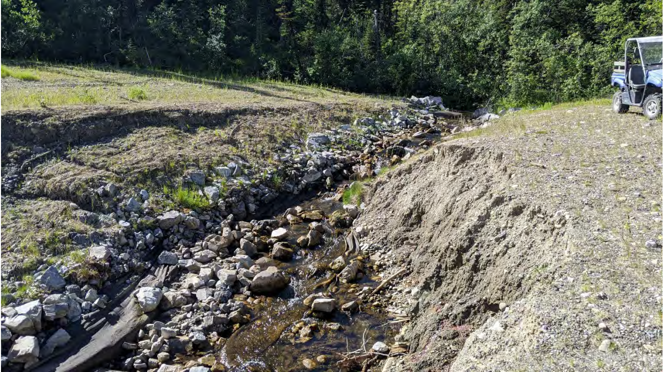
Photo NC-01: Channel Erosion at North Creek across the decommissioned access road to Burnick Zone.
