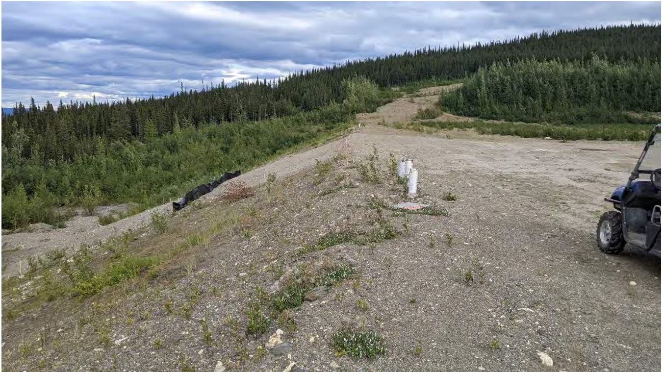
Photo ND-01: North Dam looking east towards the erosion gully repair area.
