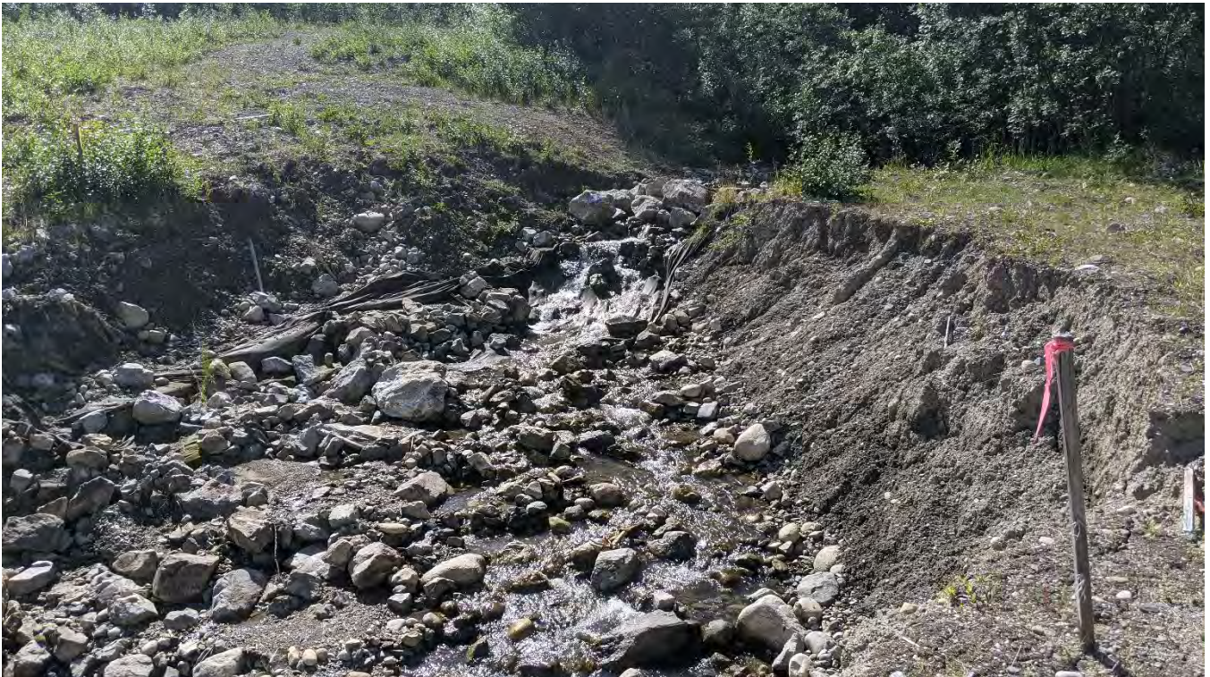
Photo NC-06: On-going channel and bank erosion at the upstream end of the lower decommissioned access road crossing of North Creek to the landfill area.
