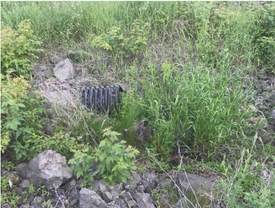
Photo II-40 Outlet of 460 mm culvert on north bank of Ed Creek Diversion Channel
