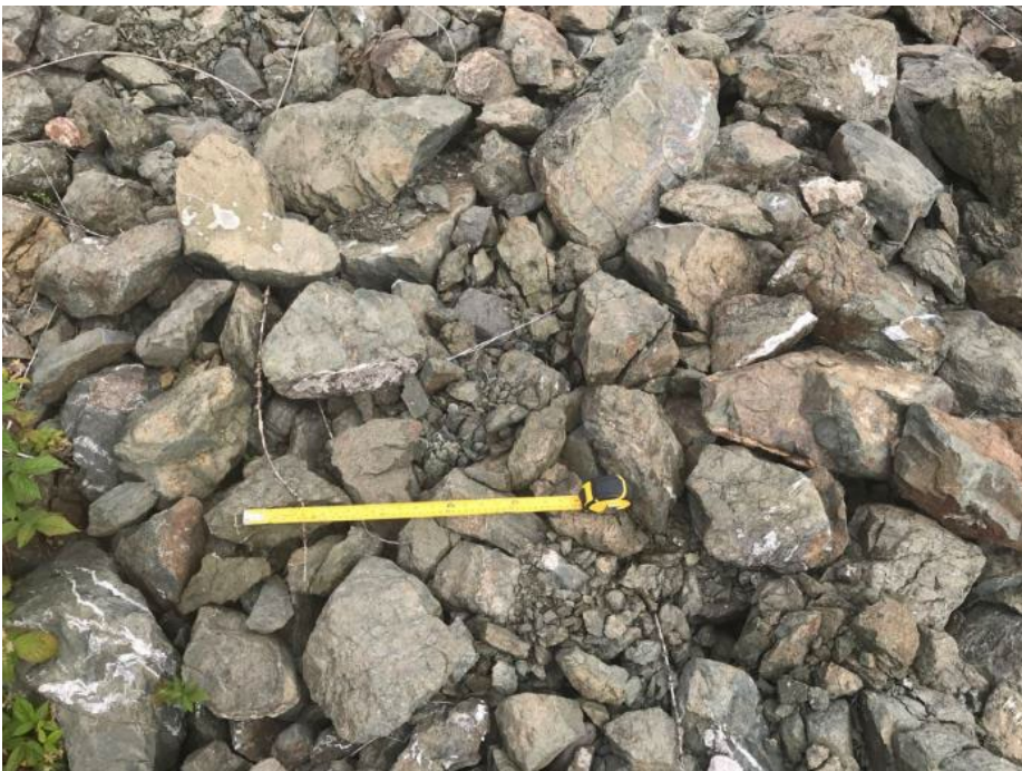
Photo II-36 Ed Creek Diversion Channel – Riprap on right bank, showing weathering and breakage
