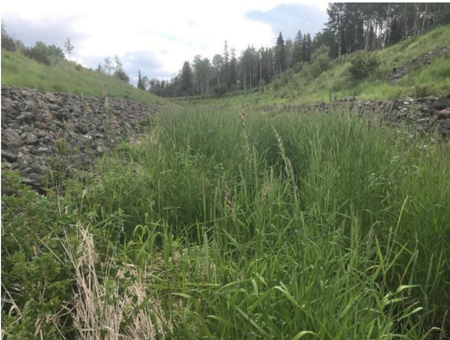
Photo II-34 Ed Creek Diversion Channel – Vegetation in channel, looking upstream from between second and third bends
