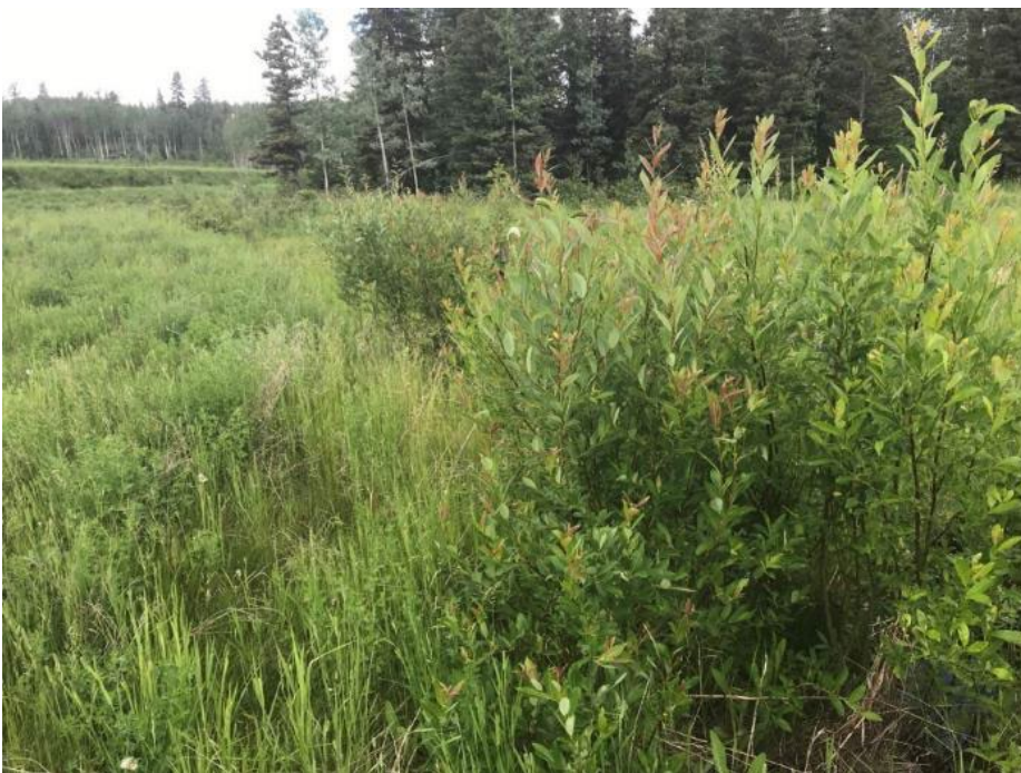
Photo II-42 Ed Creek Diversion Channel – Ditch upstream of culvert inlet and Ed Creek Diversion Channel
