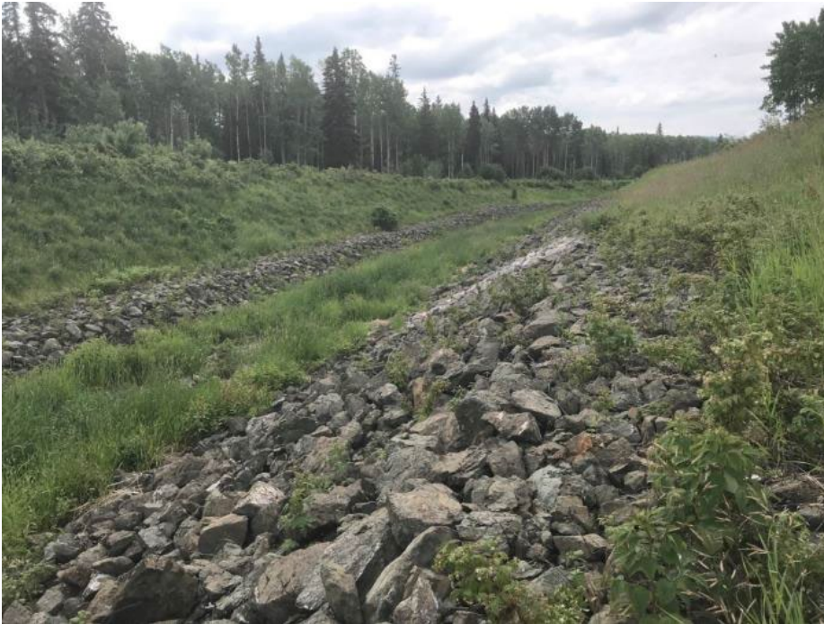
Photo II-37 Ed Creek Diversion Channel – looking downstream from between first and second bends
