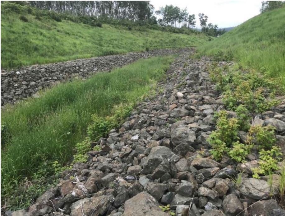
Photo II-33 Ed Creek Diversion Channel – looking downstream from between second and third bends
