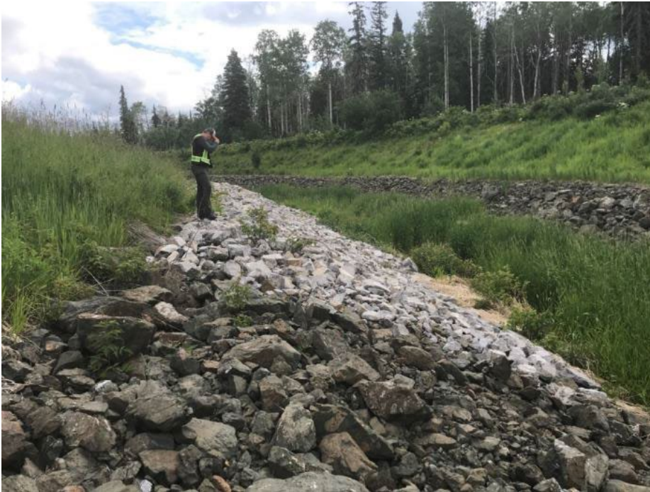
Photo II-35 Ed Creek Diversion Channel – looking upstream from near second bend. Light coloured area of riprap was replaced in 2014 and is in good condition
