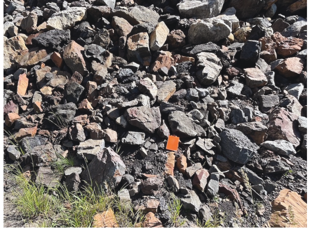
Photo 10: Riprap degradation due to weathering on several pieces of riprap (approx. Sta. 0+275)
