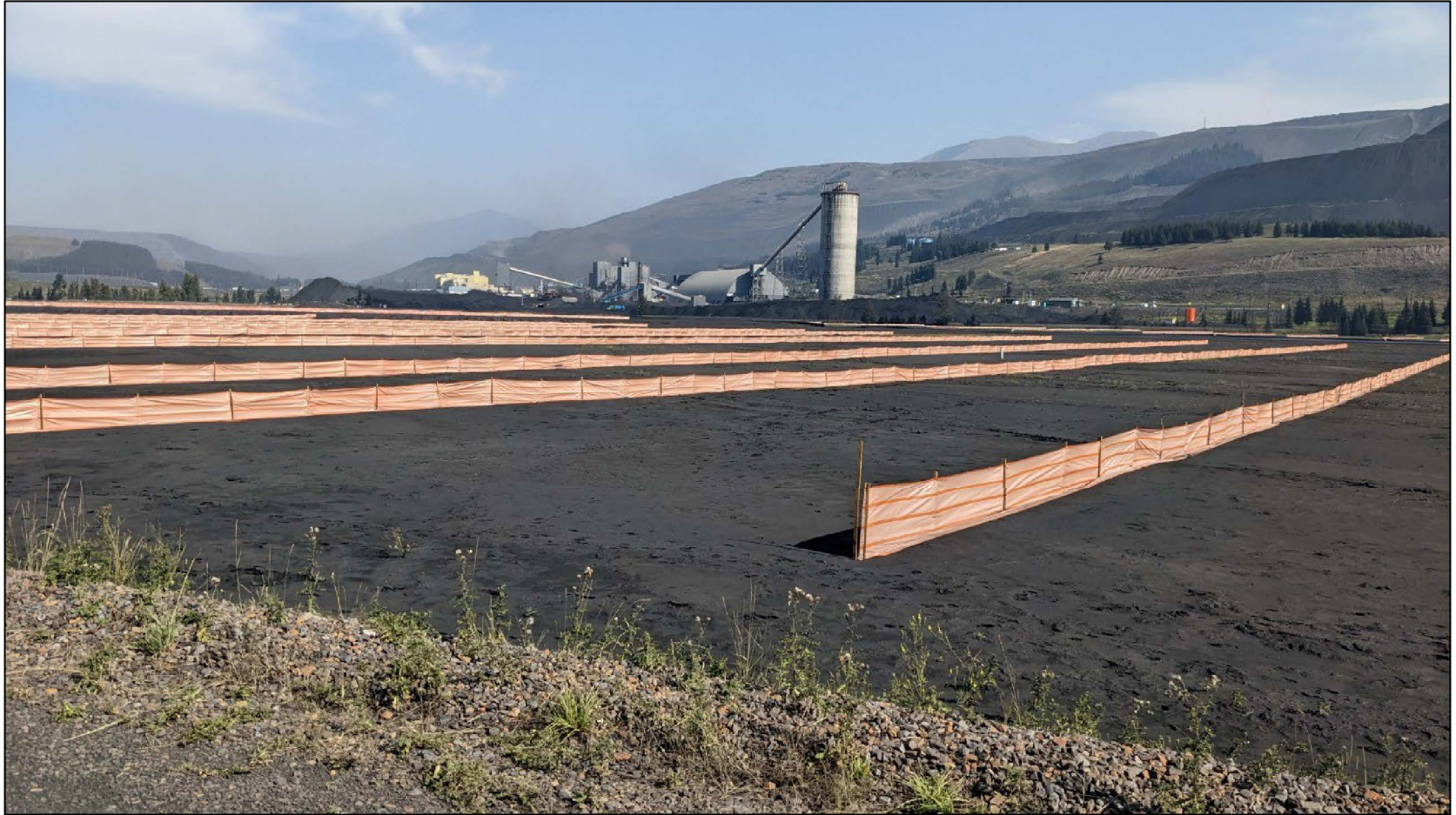
Silt fences installed at northern end of STP beach, looking northeast from approximately Sta. 0+375.
