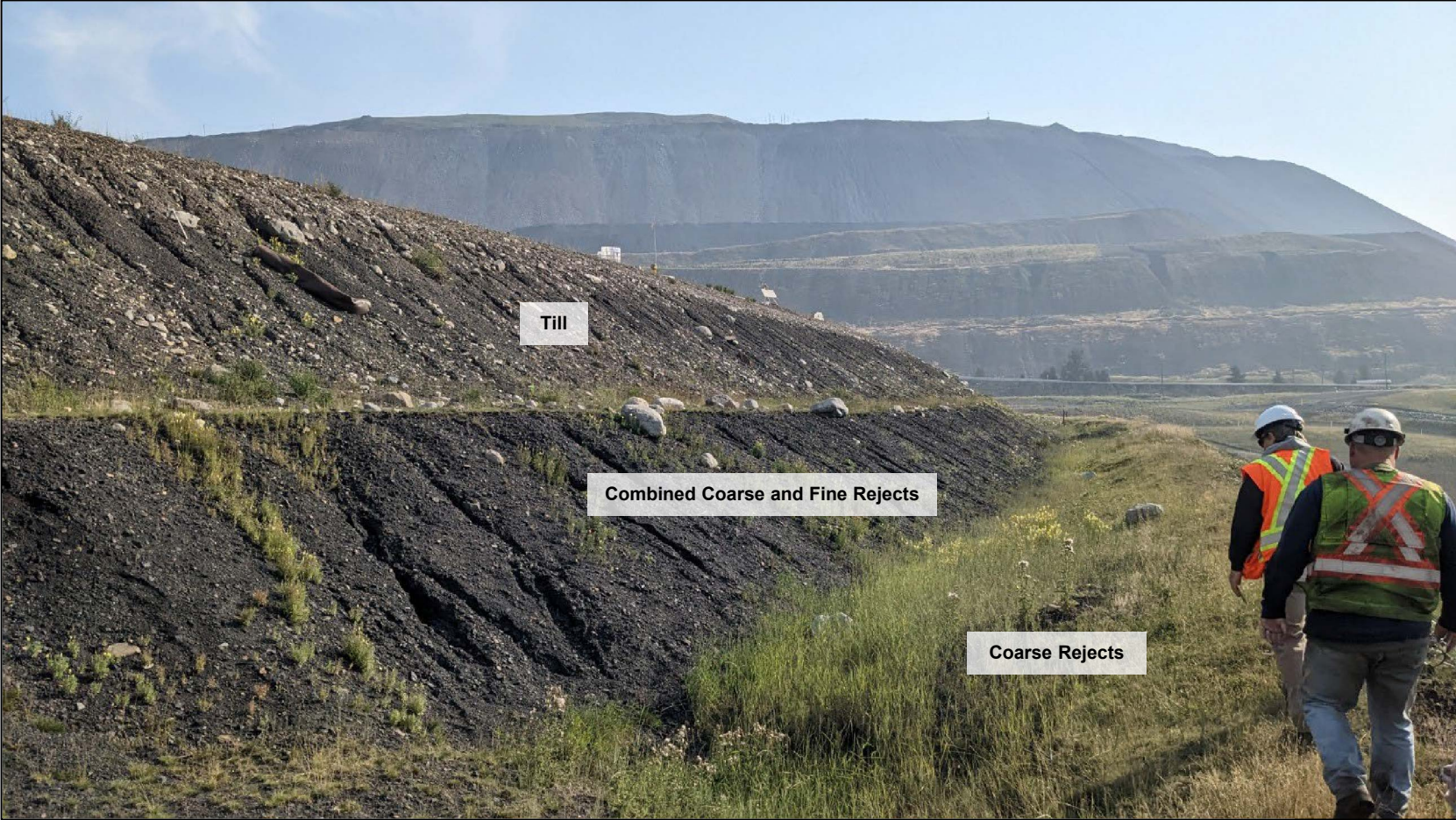
STP Main Dam downstream slope showing till, CCFR, and CR slopes, looking east from approximately Sta. 1+350.
