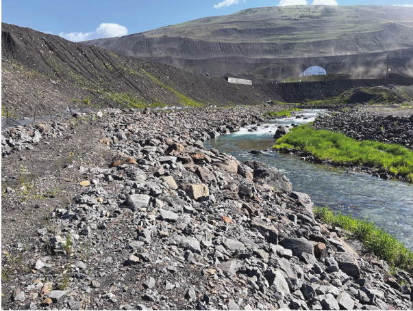
Photo 1: Looking upstream at riprap along the right bank, upstream of the NTP setback riprap.
