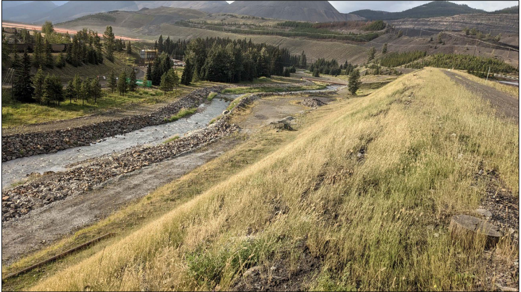
NTP Dam crest, downstream slope, and riprap along Fording River, looking southwest from approximately Sta. 1+050.
