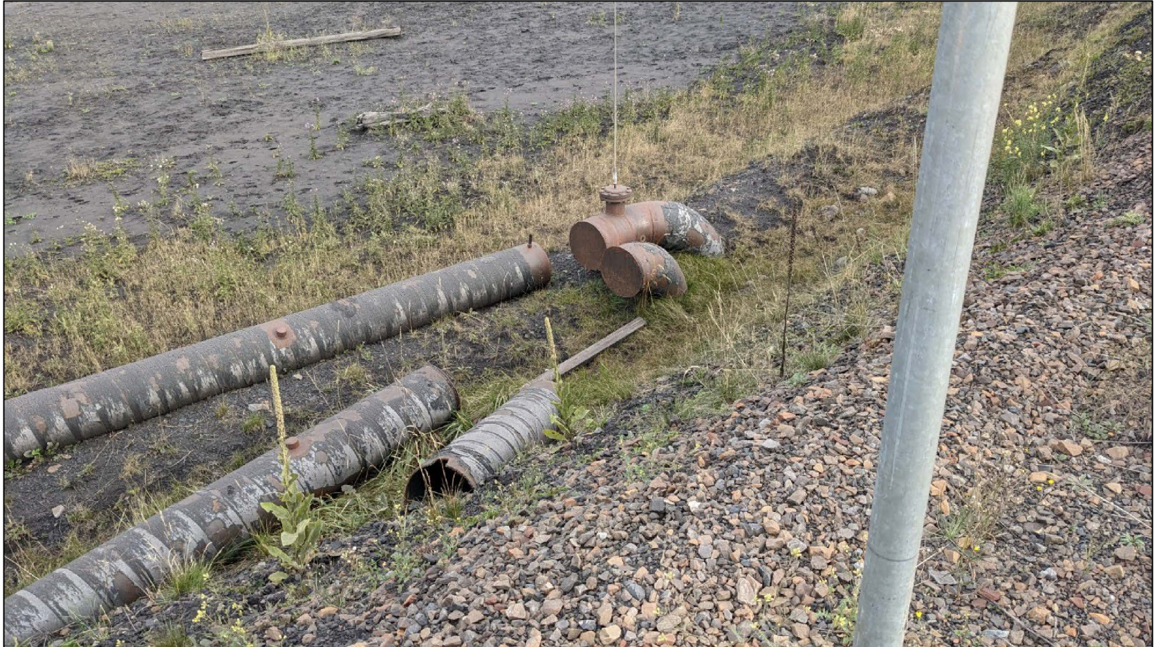
NTP capped and unused dual reclaim pipes on upstream slope and crossing under crest, looking northwest from approximately Sta. 0+850.
