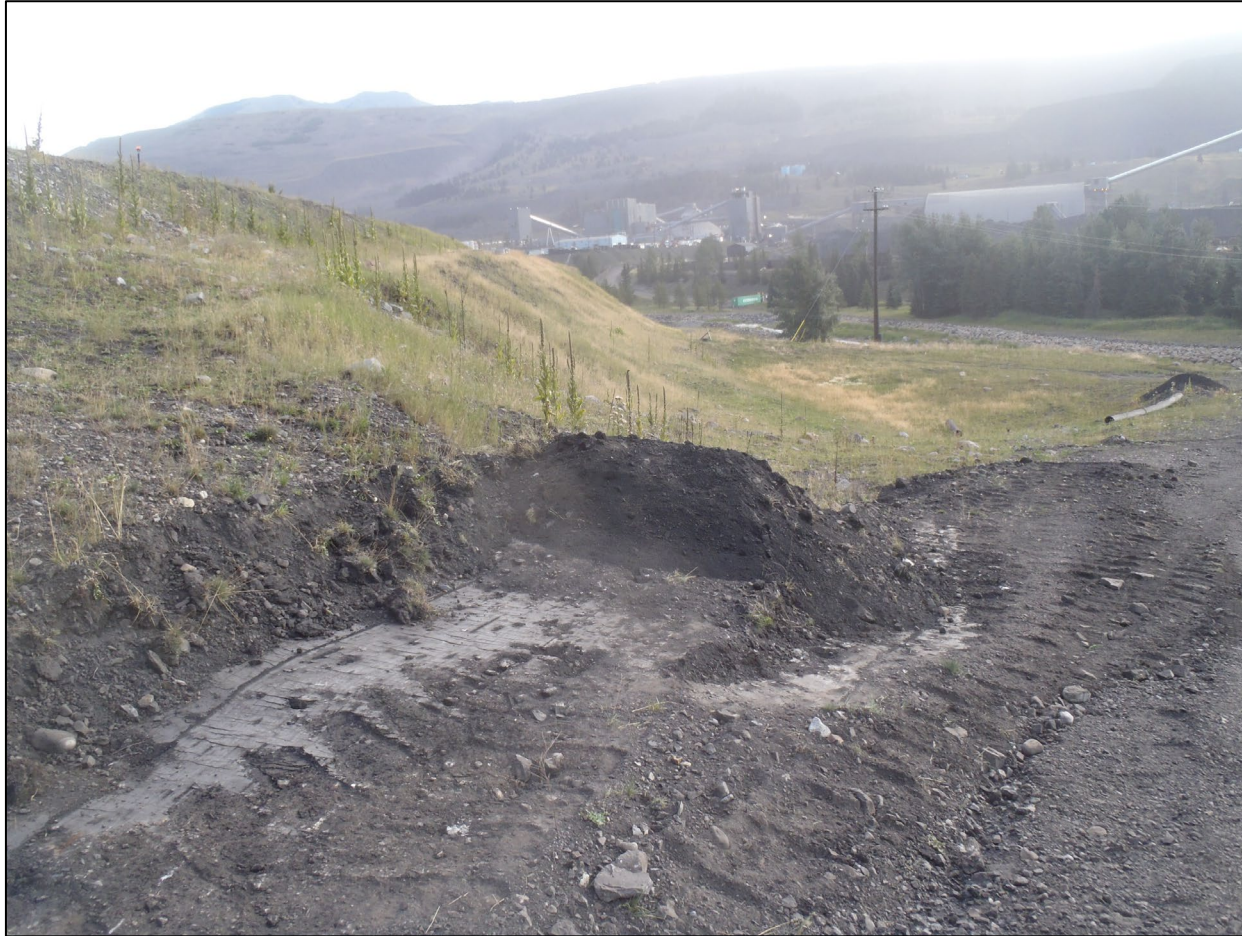
NTP Dam downstream slope and toe, damage from heavy equipment, looking northeast from approximately Sta. 1+375.
