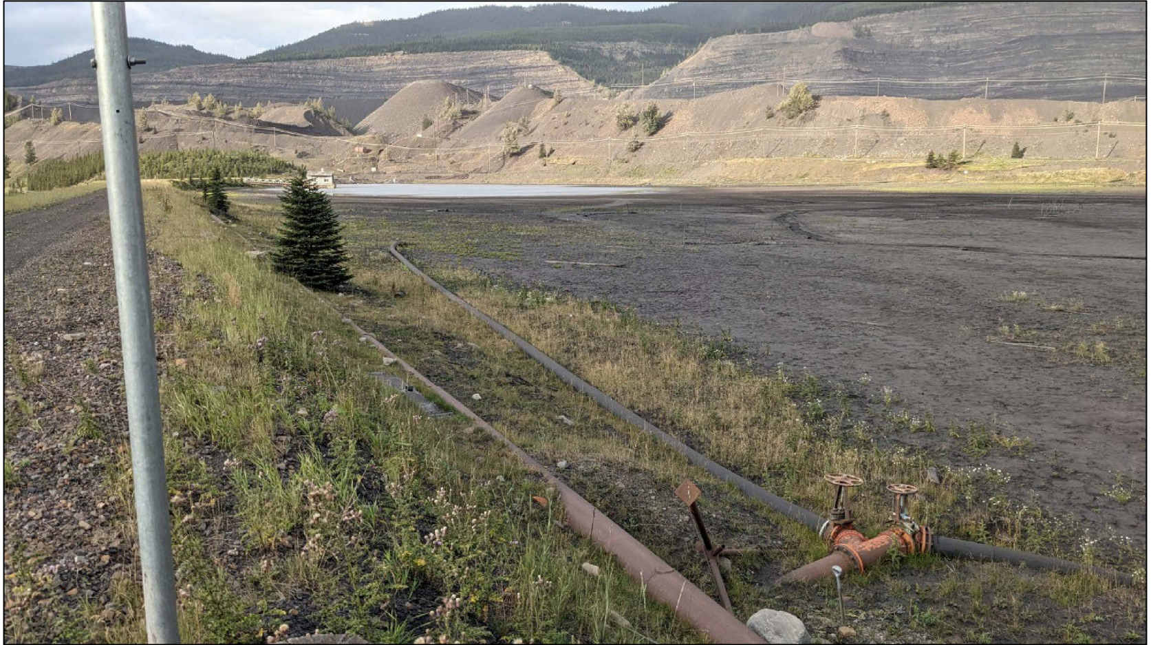
NTP Dam crest, upstream slope, and tailings surface, steel pipe runs under dam crest valves observed to be closed, looking southwest from approximately Sta. 0+950.
