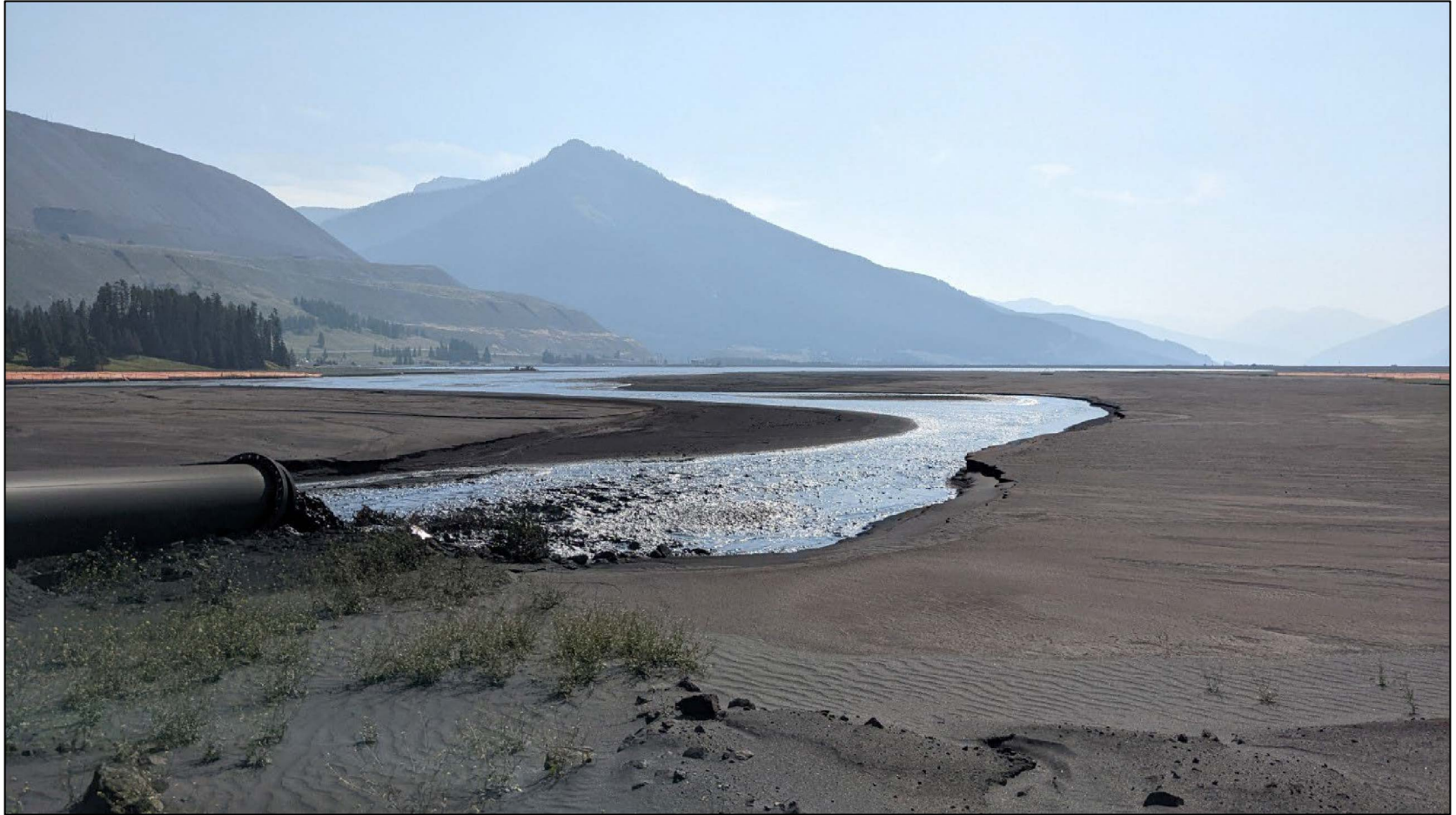
STP tailings pipeline at north single point discharge, north beach area, looking southeast.
