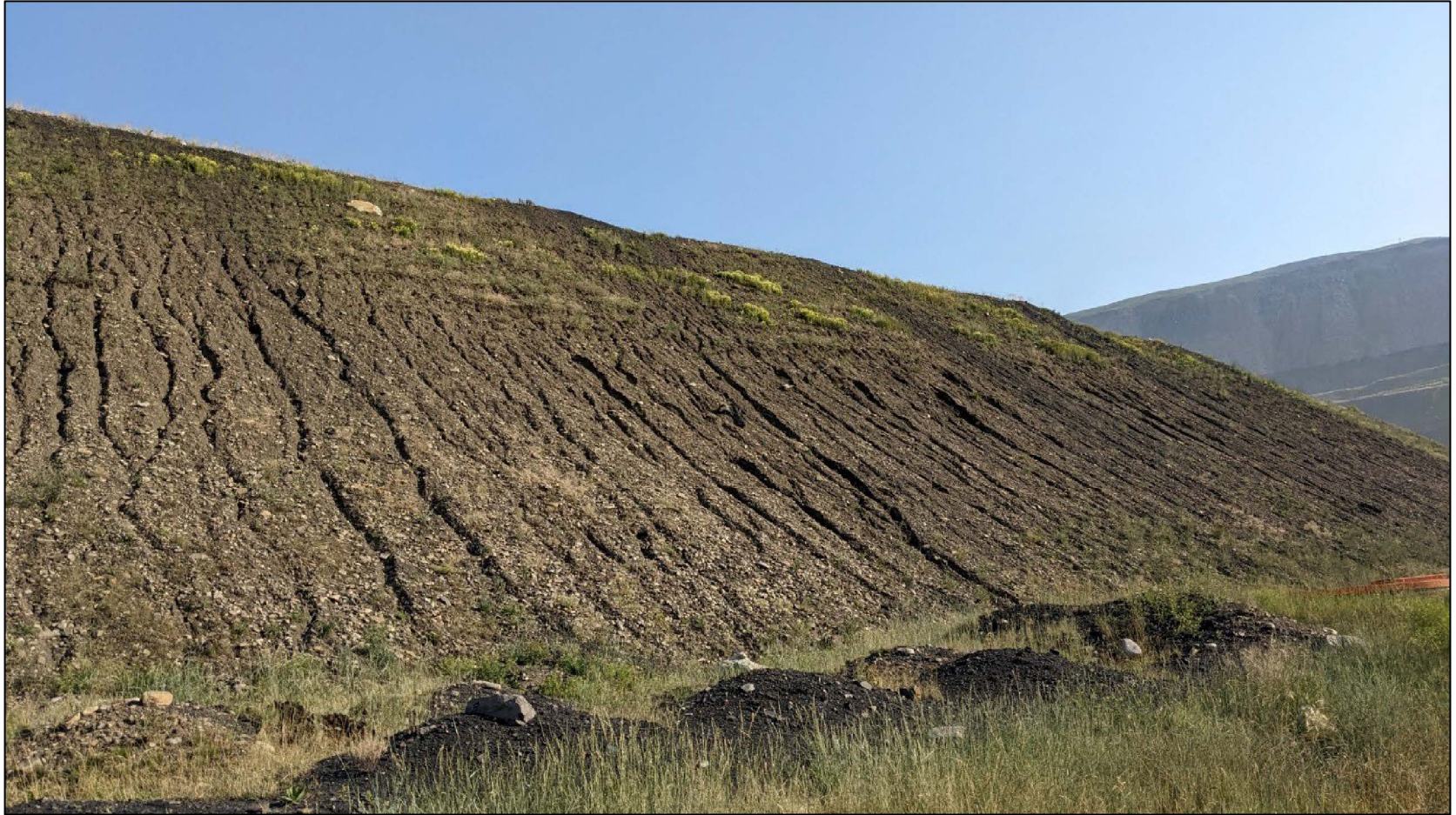
STP Main Dam downstream slope showing surficial erosion, looking northeast from approximately Sta. 1+375.
