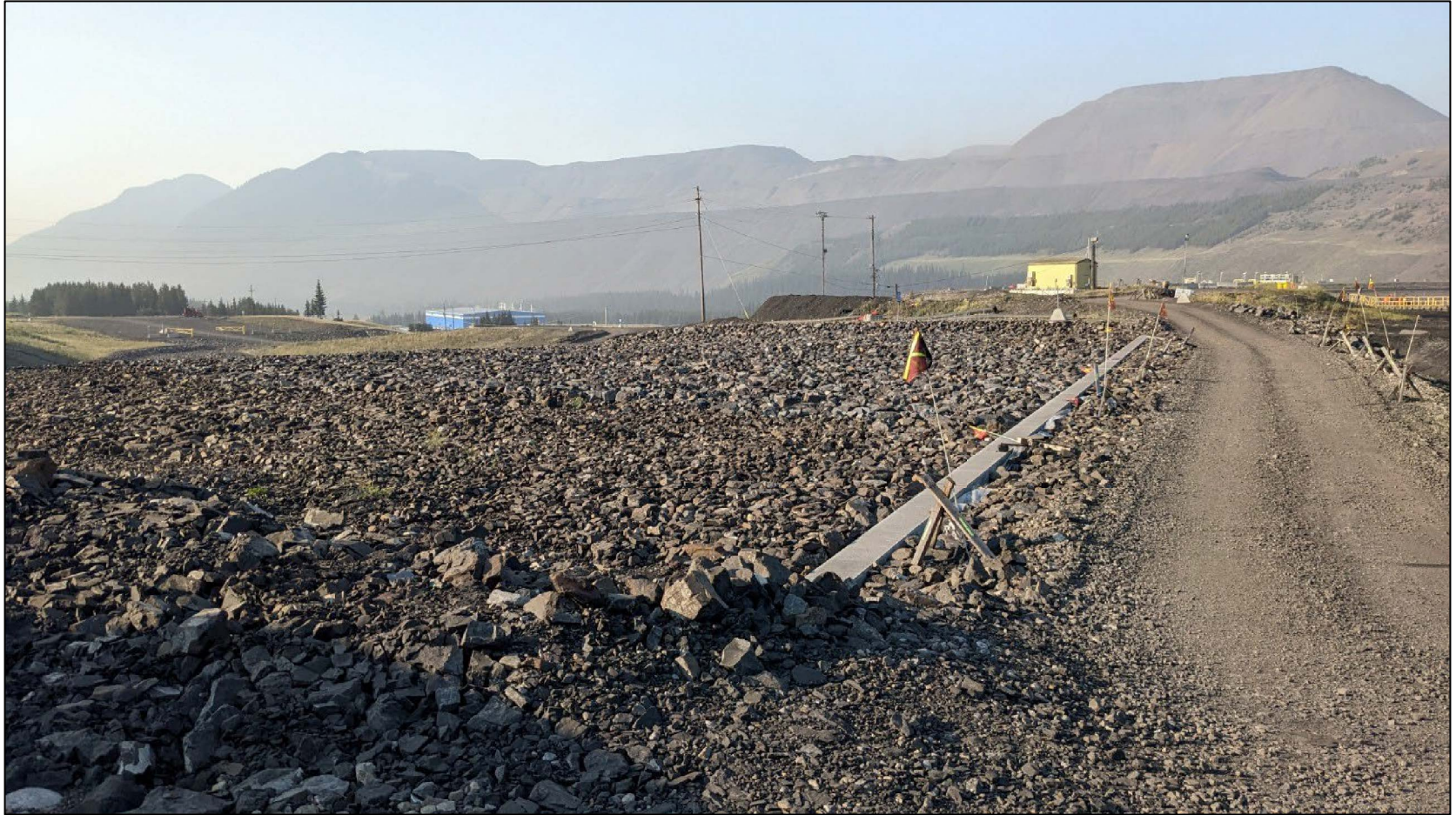
STP spillway channel and concrete sill at invert, looking southwest from STP south abutment.
