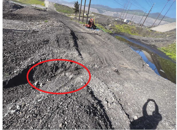
Photo 2: Riprap exposed where NTP Sumps spill from one cell to the next across the setback riprap.
