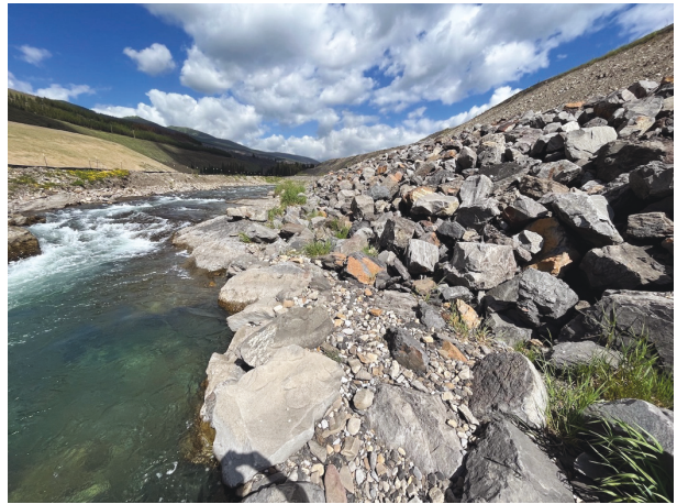
Photo 12: Erosion along the toe apron of the STP riprap at Sta. 0+670 remains the same as 2021
