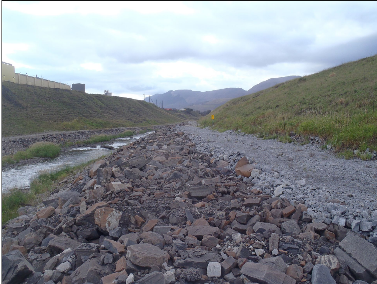
NTP Dam downstream slope and riprap along Fording River, looking southwest from approximately Sta. 0+475.
