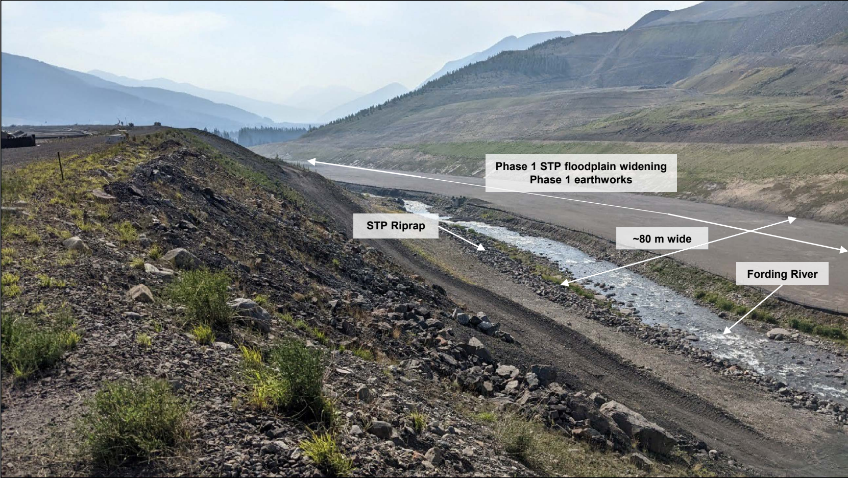
STP West Dam downstream slope, along Fording River, and widened floodplain, looking southwest from approximately Sta. 0+550.
