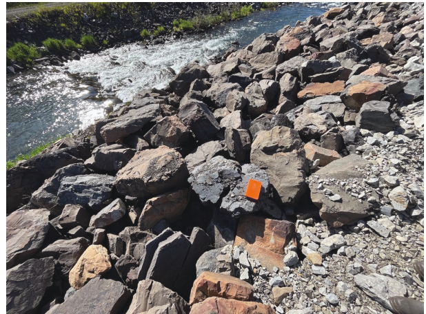
Photo 4: Riprap degradation due to weathering on several pieces of riprap (approx. Sta. 0+550)
