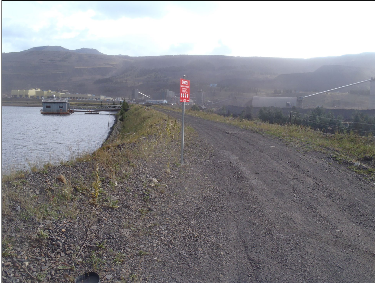
NTP Dam upstream slope and crest at south end, looking northeast from approximately Sta. 1+350.
