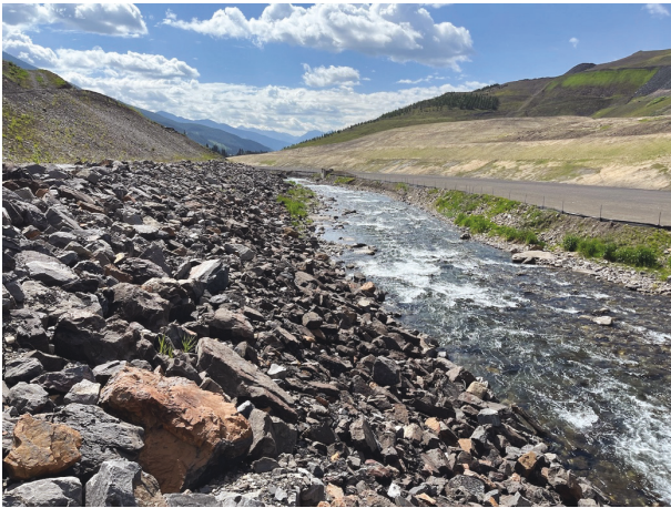
Photo 11: Looking downstream at STP riprap (from approx. Sta. 0+600). The right bank has been excavated/widened and the pipe bridge removed
