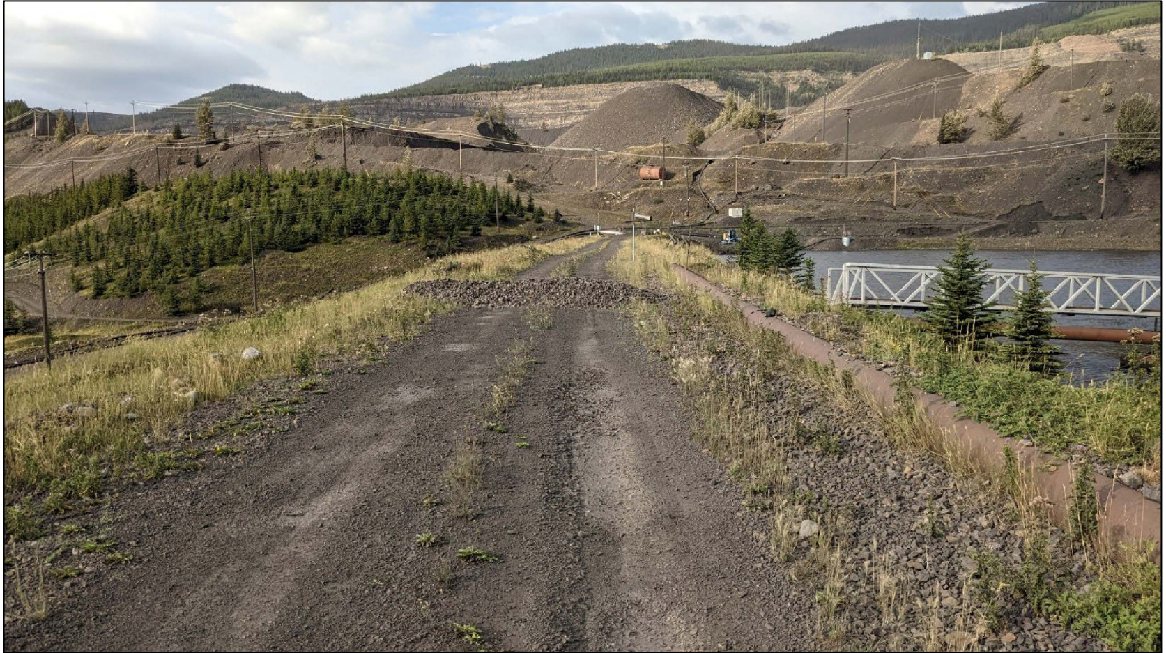
NTP Dam crest with temporary berm placed on crest, looking southwest from approximately Sta. 1+225.
