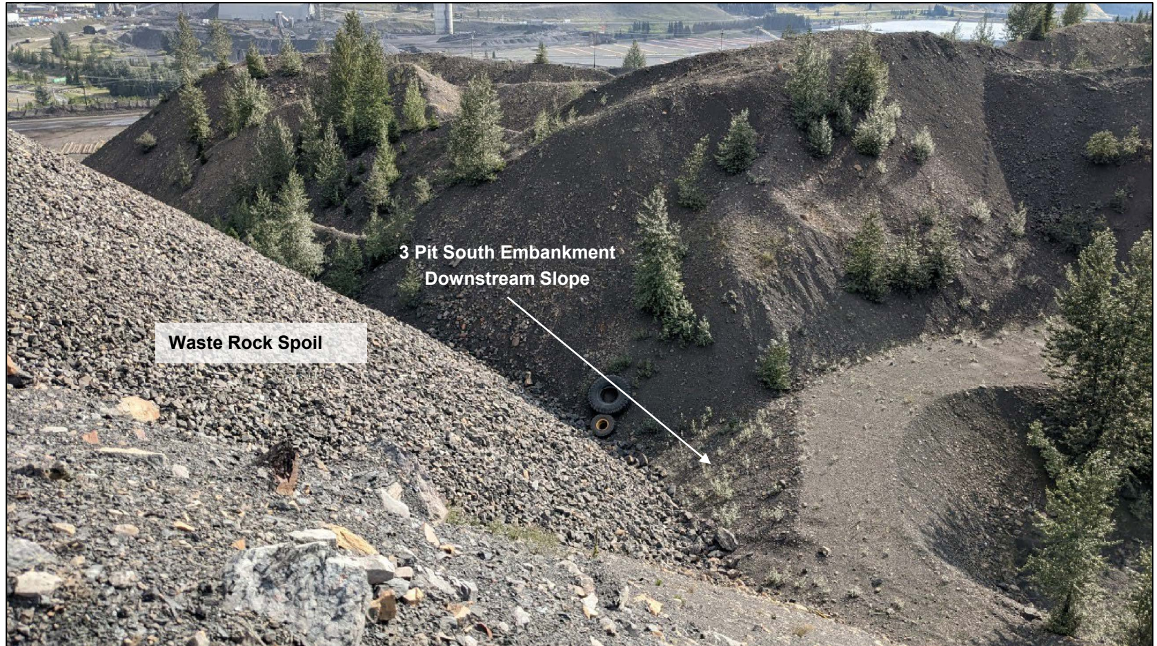
3 Pit South downstream slope, partially filled with adjacent spoil expansion, looking east.
