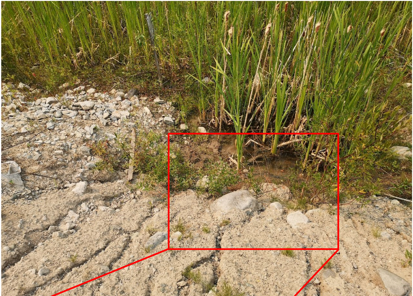
Photo I-B-35 S5 Pond: Spillway Overflow pipes partially blocked at intake by sand bags. Potential animal burrow identified. KCB suggests clearing out vegetation from spillway channel and backfilling potential animal burrow (HGH-2021-36 and HGH-2021-37).
