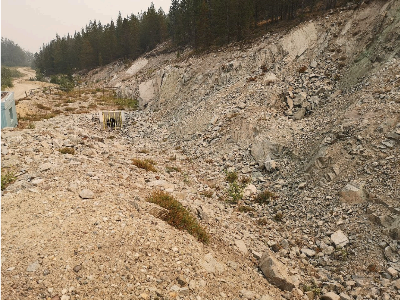
Photo I-B-5 S1 Pond: Spillway channel and pipe intake looking downstream. Channel is clear of vegetation and no sign of obstruction was observed at the pipe intake (HGH-2021-18).
