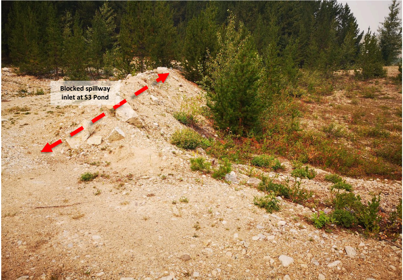
Photo I-B-25 S3 Pond: View of blocked spillway inlet at right abutment (HGH-2021-30).
