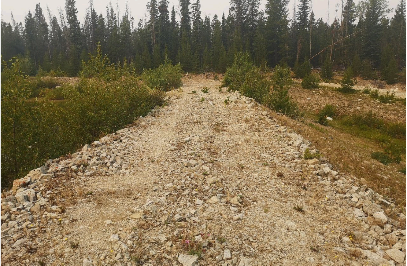
Photo I-B-8 S2 Pond: View of S2 Pond embankment crest, view from mid dam towards left abutment (HGH-2021-22).
