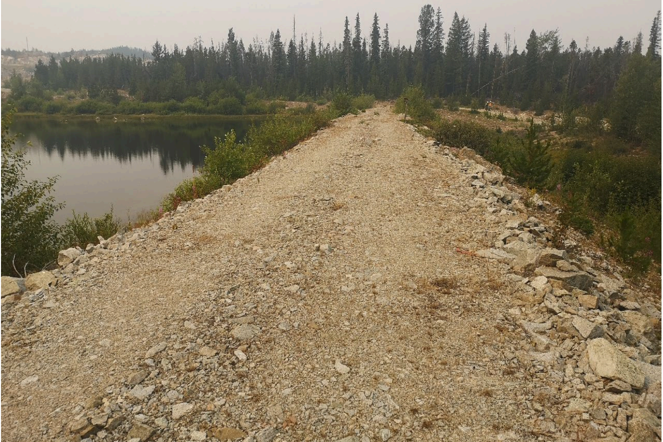
Photo I-B-7 S2 Pond: View of S2 Pond embankment crest, looking toward left abutment (HGH-2021-21).
