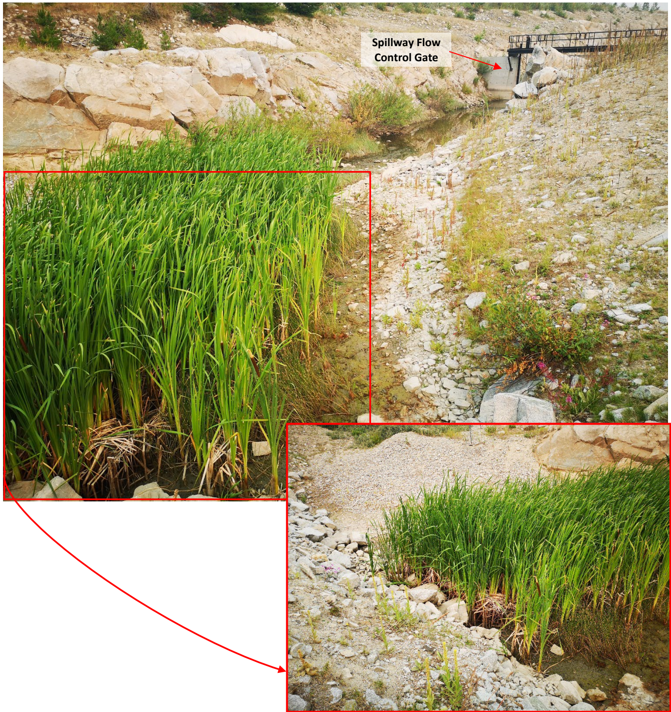
Photo I-A-20 Area downstream of approach channel culverts and upstream of flow control gate – Culverts and channel were partially obstructed during the site visit, but vegetation was cleared by HVC in Q3/Q4 2021 as part of routine maintenance (HGH-2021-11)
