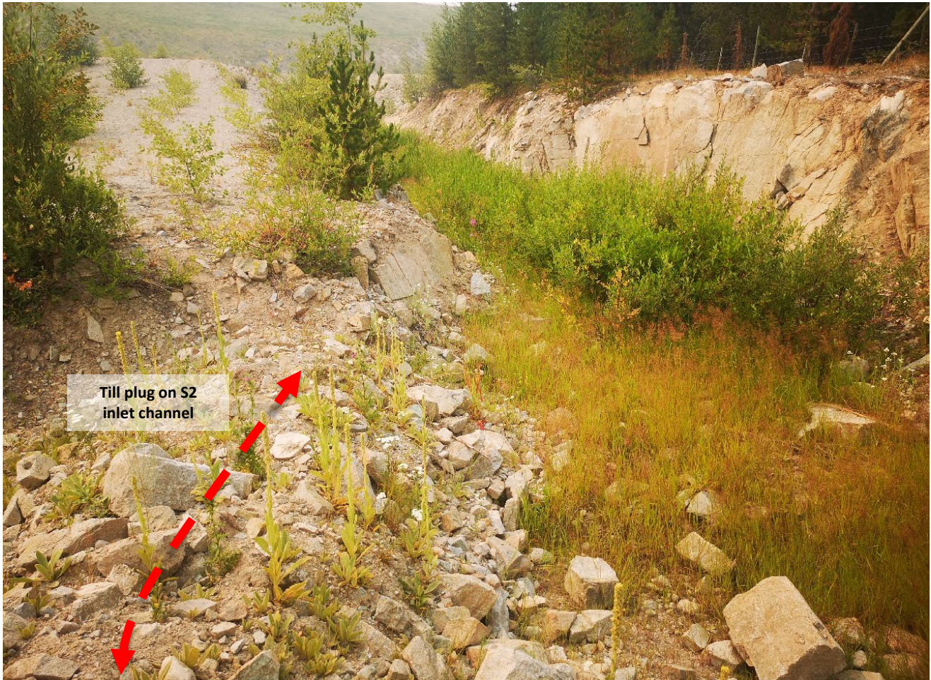
Photo I-B-13 S2 Pond: Till plug (~1.2 m high and ~ 1m wide) is placed in S2 inlet channel. Highmont TSF Spillway diversion channel is heavily vegetated; needs to be cleared as part of routine maintenance (HGH-2021-24).
