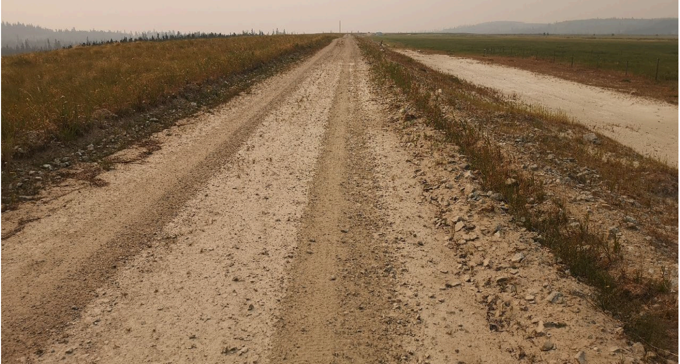
Photo I-A-7 East Dam crest. Crest is in good condition. No signs of deformation or distress were observed (HGH-2021-02)
