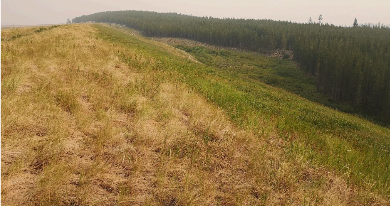
Photo I-A-11 East Dam downstream slope. Slope is vegetated and in good condition (HGH-2021-07)
