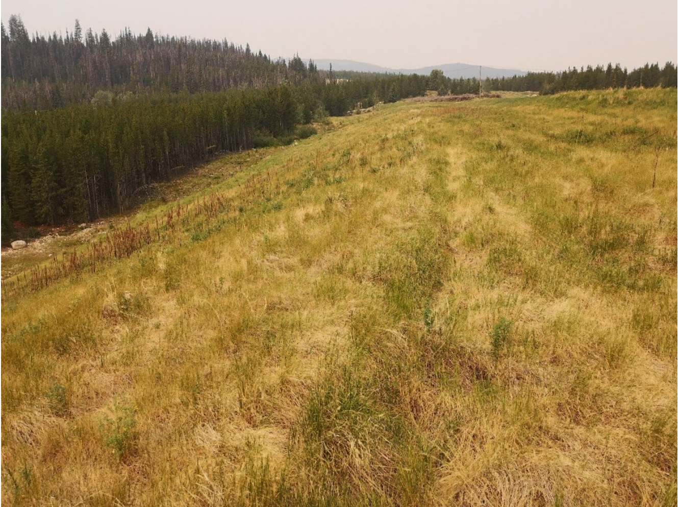
Photo I-A-17 View of South Dam downstream slope at right abutment looking northwest. Slope is vegetated and in good condition (HGH-2021-09)
