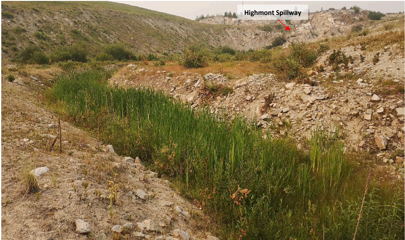
Photo I-A-28 North Dam downstream slope and toe, downstream of Highmont Spillway. North dam toe is in good condition. Spillway stilling basin is heavily vegetated. (HGH-2021-16)
