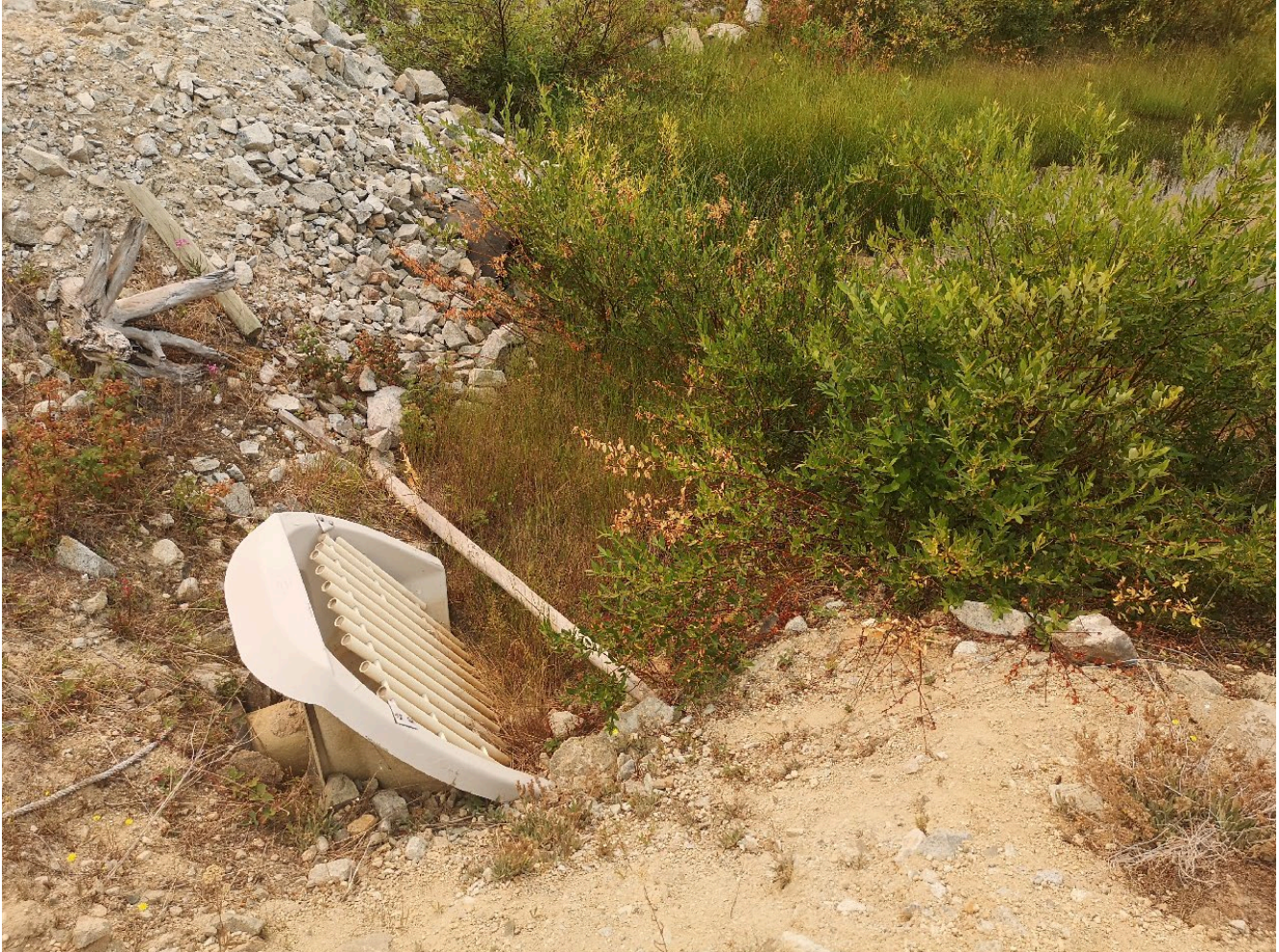
Photo I-B-42 S8 Pond: Overview of overflow pipe trash rack. Rack is clear of debris. Current water level is below the invert (HGH-2021-40).
