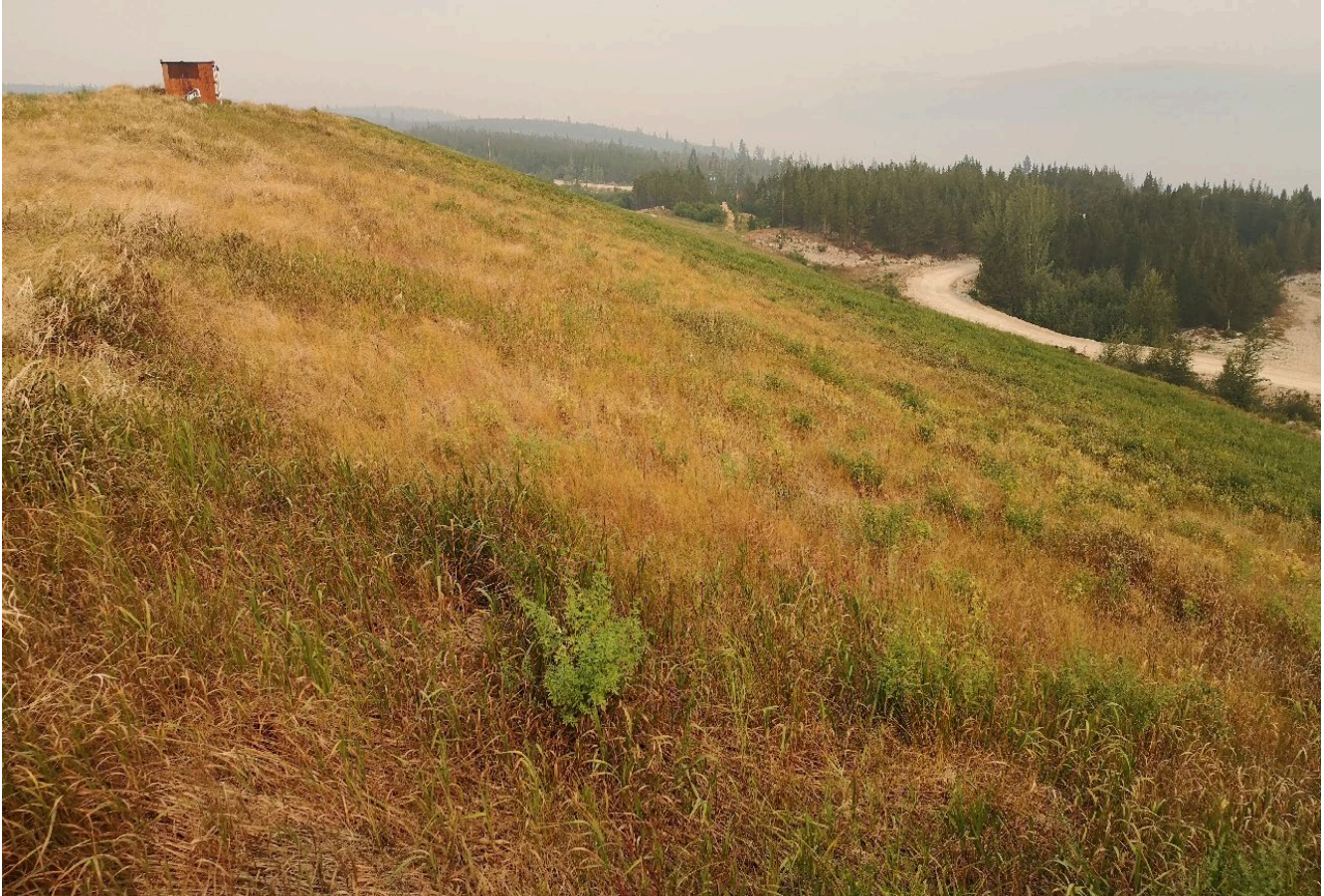
Photo I-A-8 View of North Dam downstream slope looking northwest. Vegetation was about 0.5 m tall. No signs of distress or deformation were observed (HGH-2021-06)
