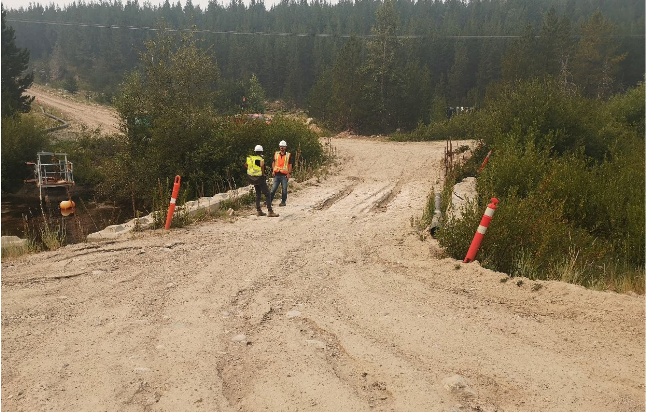
Photo I-B-27 S5 Pond: View of access road on the divider dyke. Minor rutting observed on crest of divider dyke is managed under routine maintenance (HGH-2021-31).
