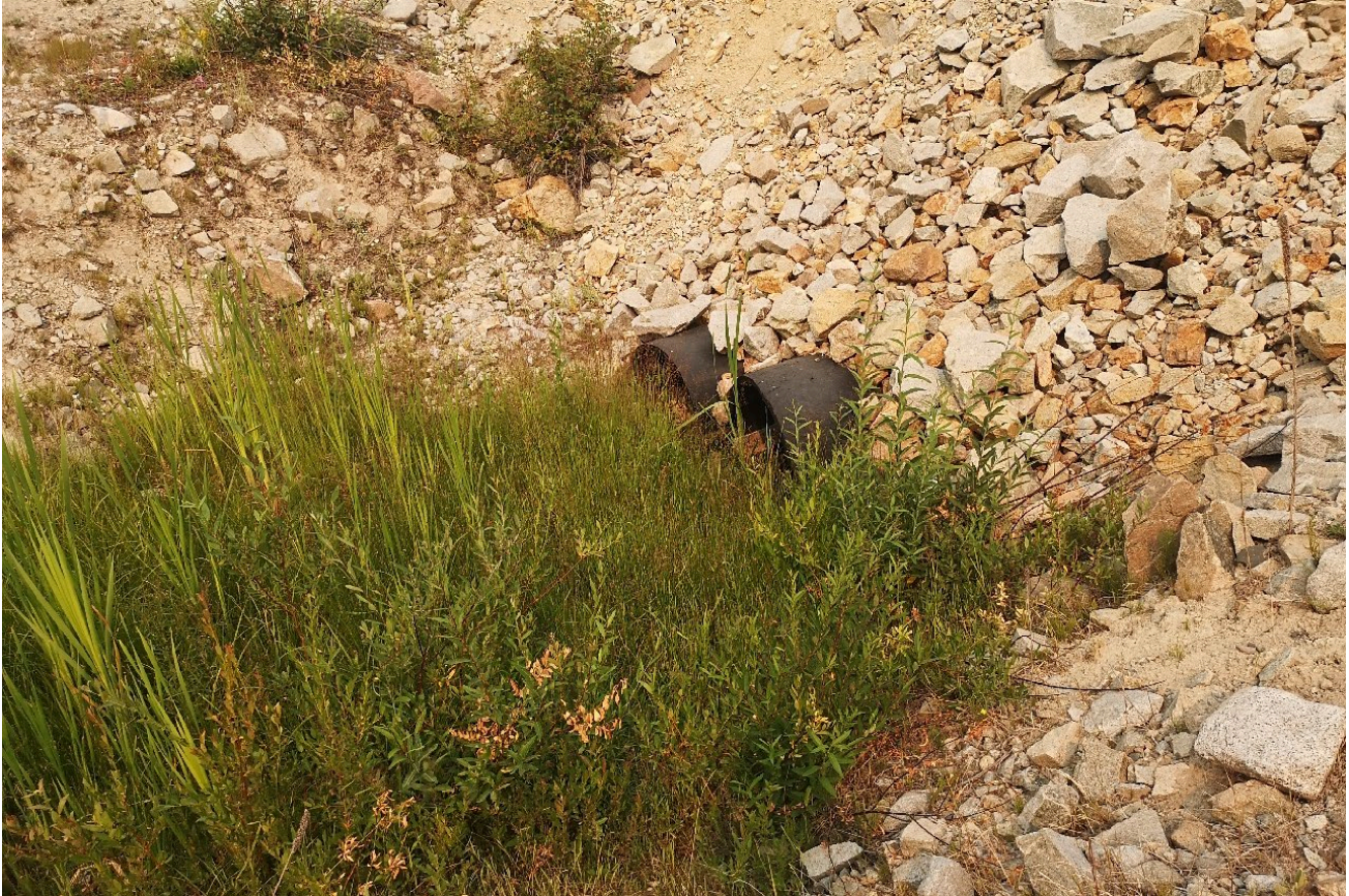
Photo I-A-30 North Dam toe access road crossing culverts. Culverts are misshapen; see AFPR recommendation HD-2017-01 (HGH-2021-16)
