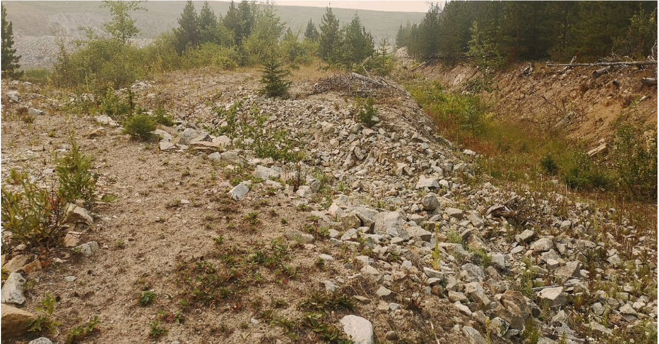
Photo I-B-15 S2 Pond: View of Highmont Spillway channel. Channel is in good condition. Excess vegetation needs to be removed by HVC as part of routine maintenance (HGH-2021-25).
