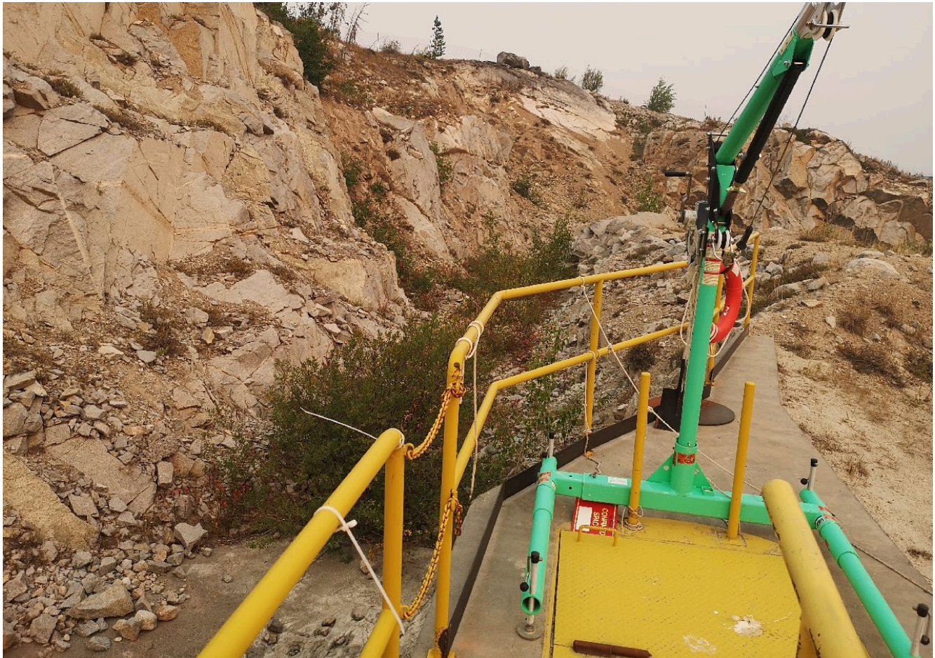
Photo I-A-25 Highmont Spillway channel, downstream of S1 Pond diversion and control. No flow downstream of S1 diversion. Minor vegetation was observed in the channel (HGH-2021-14)
