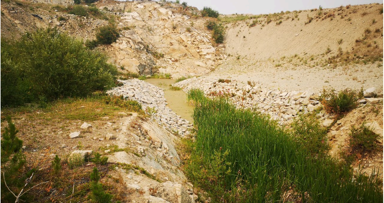
Photo I-A-29 Water is ponded downstream of spillway drop. Vegetation obstructing spillway channel (HGH-2021-17)
