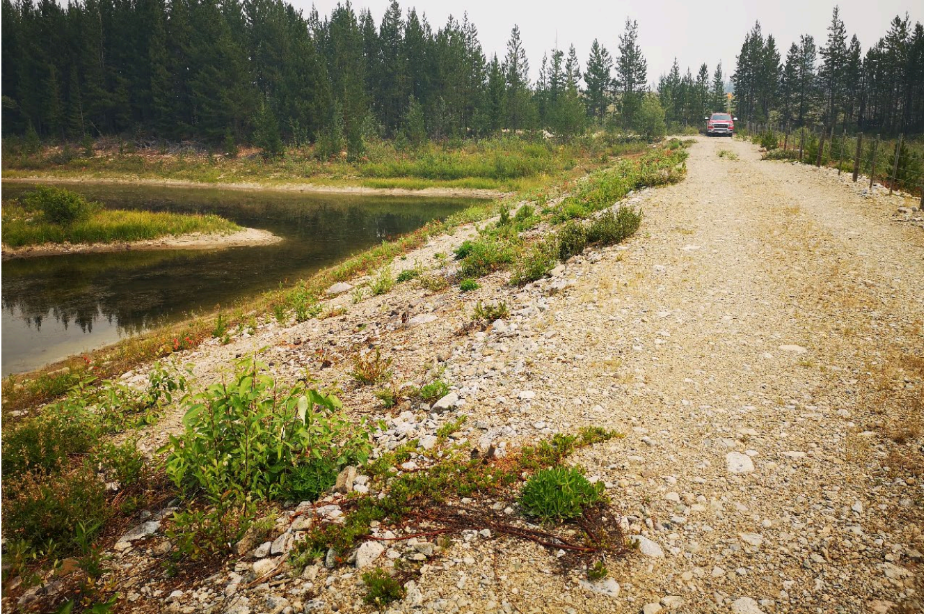
Photo I-B-18 S3 Pond: Overview of dam crest from mid dam, looking toward left abutment (HGH-2021-28).
