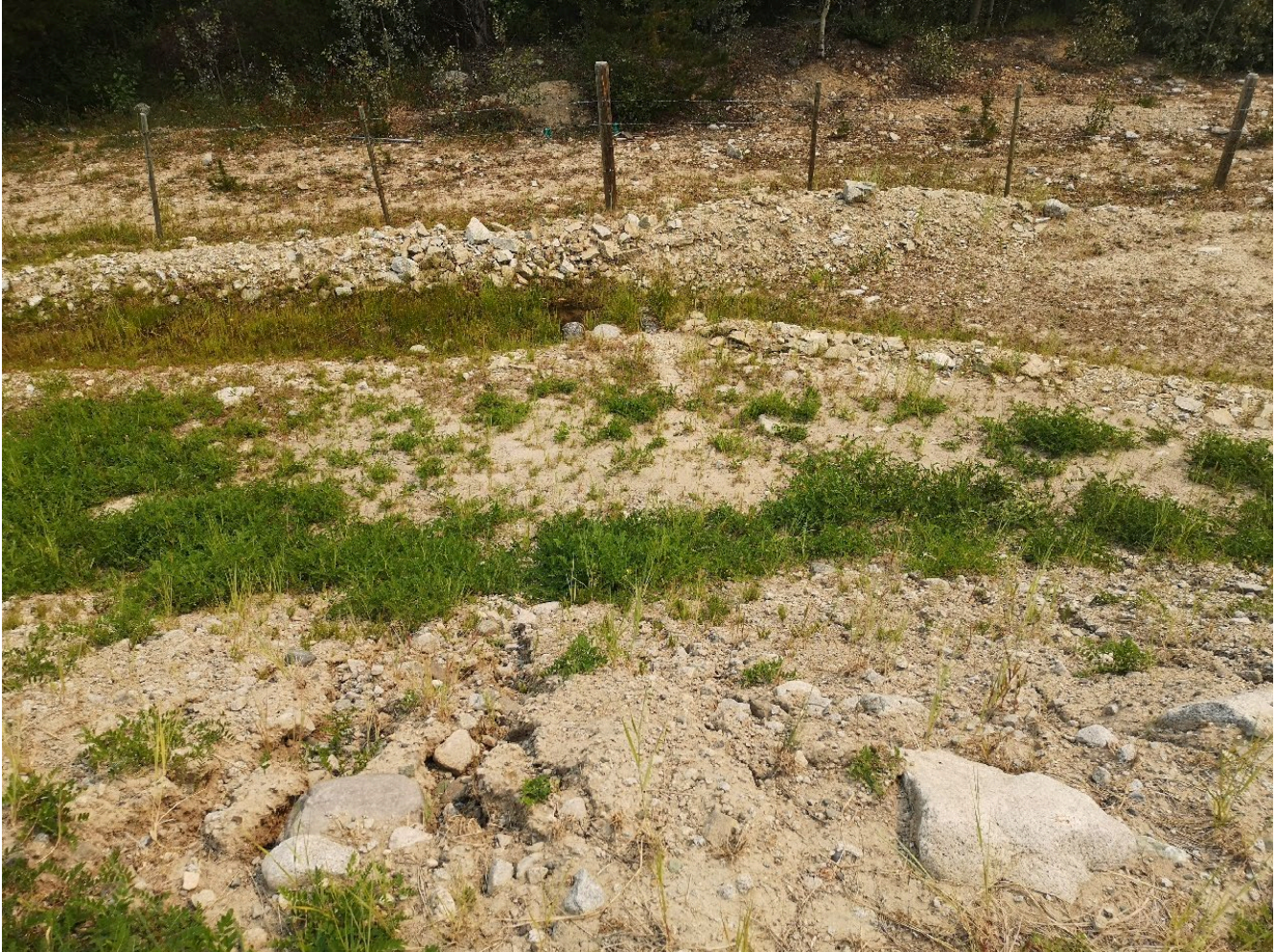
Photo I-B-36 S5 Pond: Overview of downstream slope and S5 Overflow outlet pipes daylighting at toe, looking east (HGH-2021-36).
