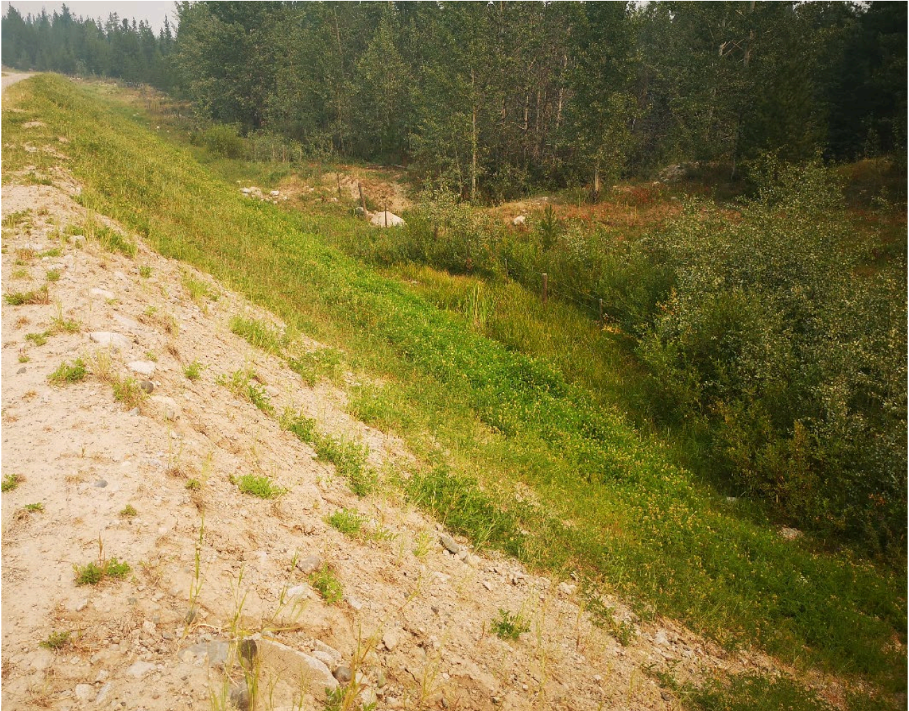
Photo I-B-37 S5 Pond: Downstream toe of perimeter crest. Change of vegetation suggests there has been temporary ponding at the toe likely due to the run-off; no signs of seepage (HGH-2021-31).
