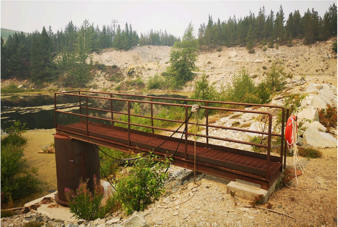
Photo I-B-4 S1 Pond: LLO to the left of spillway intake. Pond level was about 1.5 m below inlet. Vegetation partially obstructing intake; needs to be cleared during routine maintenance (HGH-2021-18).
