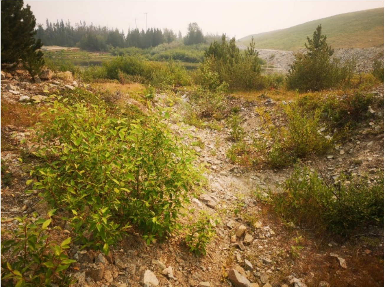
Photo I-B-14 S2 Pond: S2 Pond inlet and channel from Highmont Spillway Diversion. Channel and the inlet are vegetated; needs to be cleared as part of routine maintenance. (HGH-2021-24).
