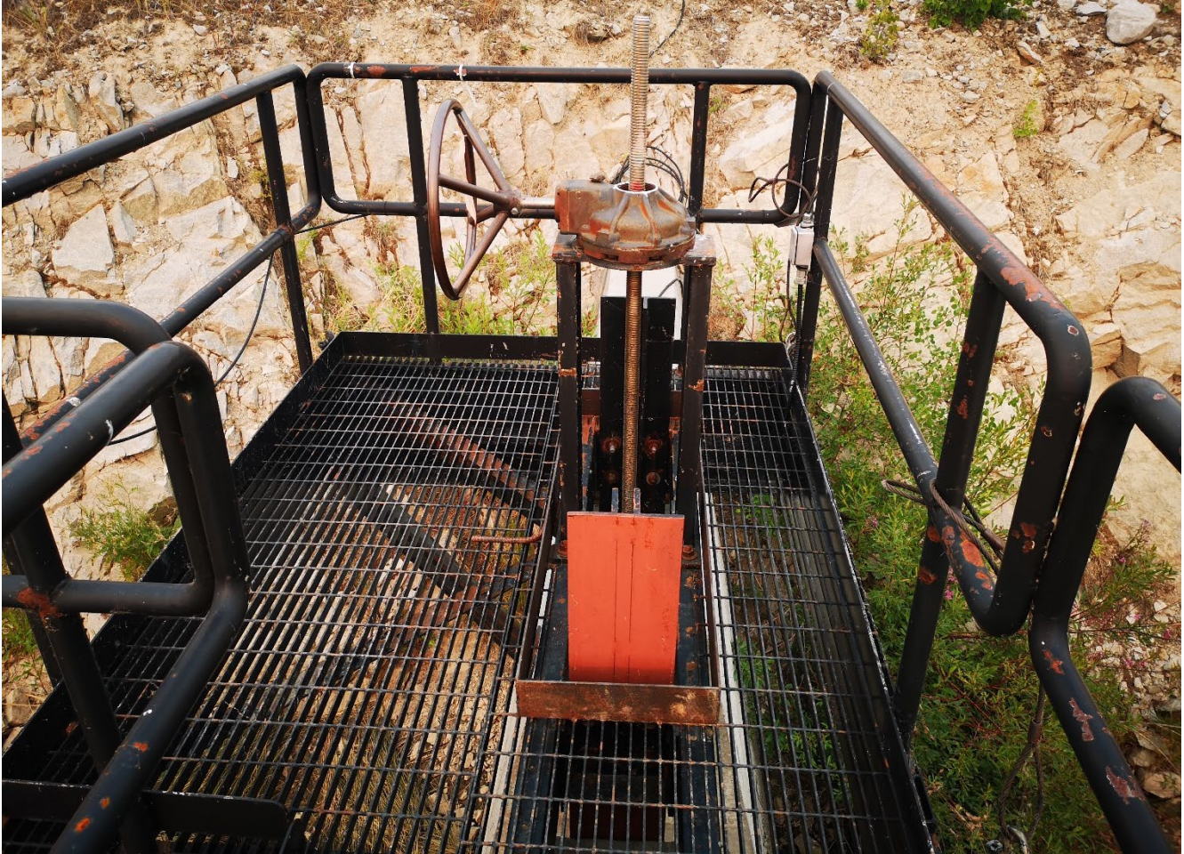
Photo I-A-21 Spillway flow control gate. Valve is operational and could move up and down (tested for slight movement). Sliding gate is slightly open (HGH-2021-12)
