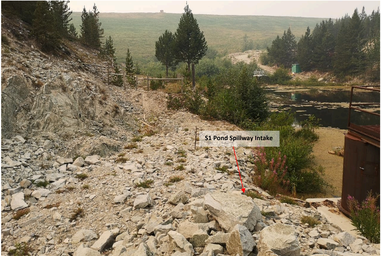
Photo I-B-3 S1 Pond: View of S1 Pond, spillway intake, and Low-Level Outlet (LLO) (HGH-2021-18).
