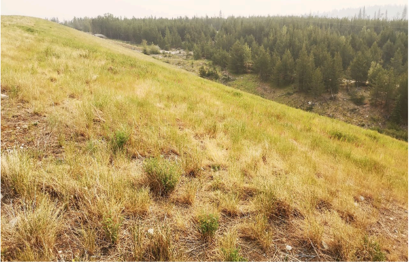
Photo I-A-12 View of South Dam downstream slope looking northeast. Slope is vegetated and in good condition (HGH-2021-08)
