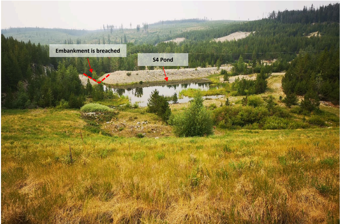
Photo I-A-16 South Dam downstream slope and view of S4 Pond from South Dam. S4 embankment is breached (HGH-2021-09)
