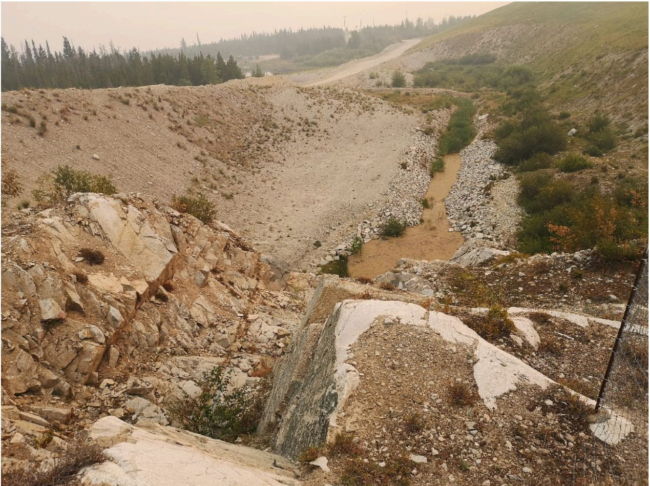
Photo I-A-27 Highmont Spillway channel downstream of spillway drop. Channel is in good condition. North Dam downstream toe is visible. No signs of distress or deformation (HGH-2021-15)
