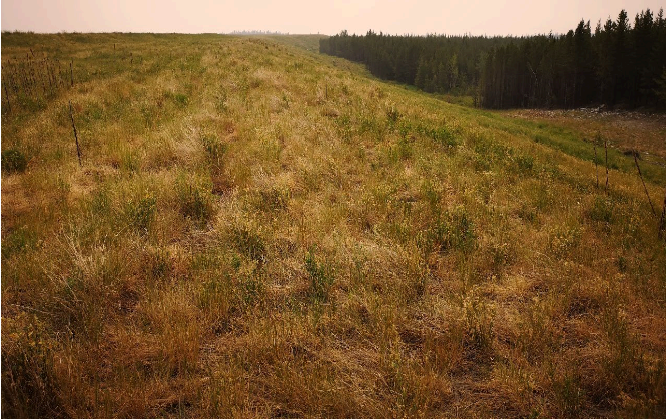
Photo I-A-15 View of South Dam downstream slope at right abutment looking east. Slope is vegetated and in good condition (HGH-2021-09)
