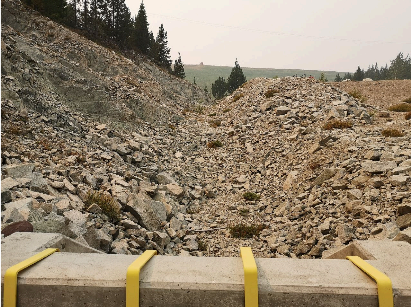
Photo I-B-6 S1 Pond: Spillway channel upstream of pipe intake, looking toward the pond (HGH-2021-20).
