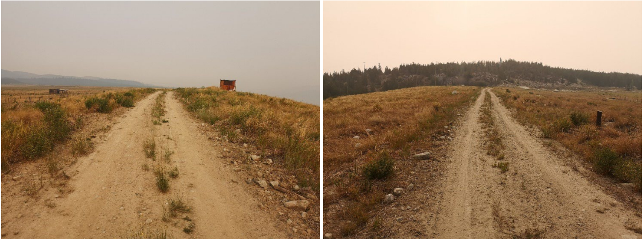
Photo I-A-6 North Dam crest near right abutment. Crest is in good condition (HGH-2021-05)
