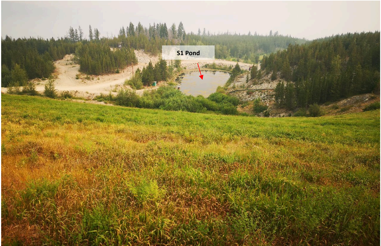
Photo I-A-9 View of North Dam downstream toe and S1 Pond. No signs of distress or deformation were observed (HGH-2021-06)
