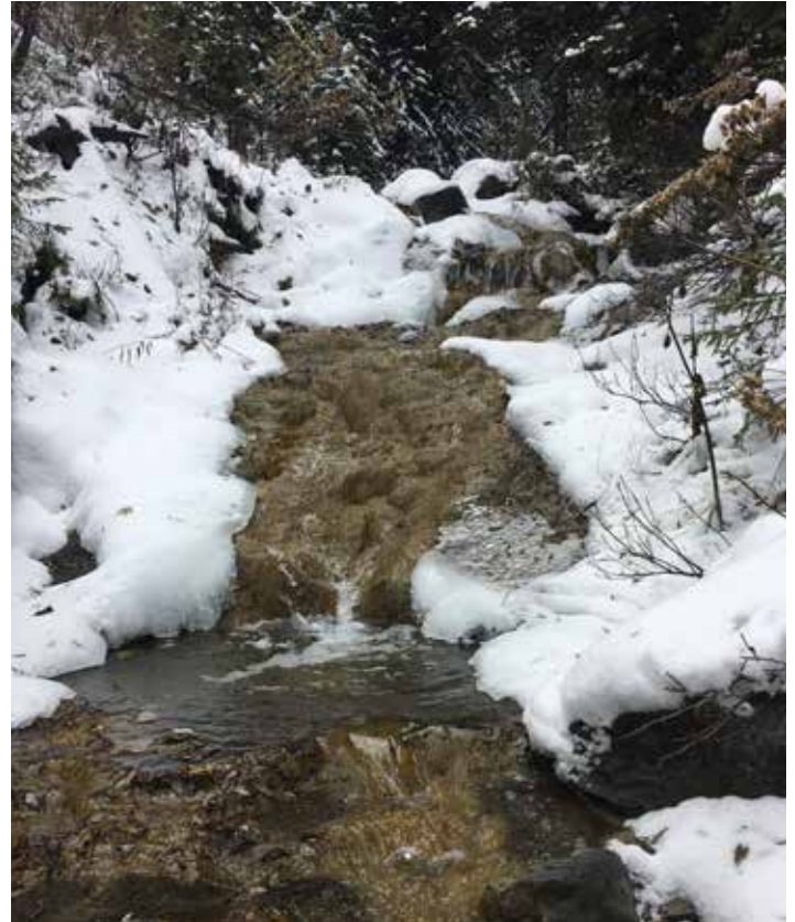
Figure 15. A fully concreted streambed in Porter Creek. This reach has a calcite index of 3.
